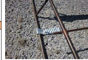
Dowel basket anchored to subgrade (upper) and existing asphalt (lower, from Maria Masten, Minnesota DOT)
