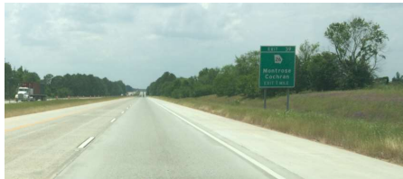
Concrete shoulders using RCA on I-16 in Georgia Photo: Georgene Geary, GGF&A
