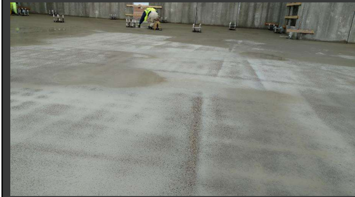
Removing Water From Surface Is Critical!
