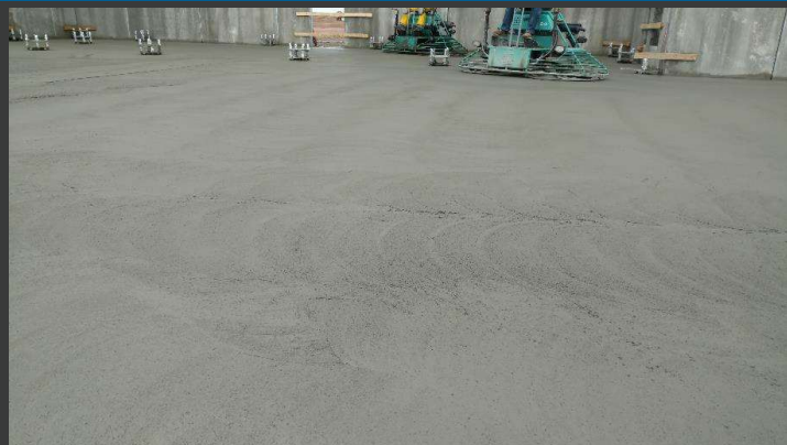
Removing Water From Surface Is Critical!
