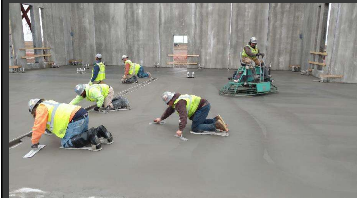
Removing Water From Surface Is Critical!
