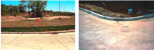
Lining joints perpendicular to pavement edge!
