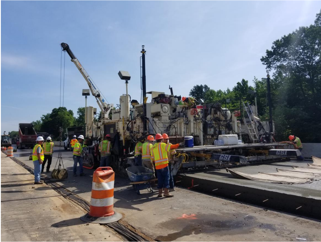
Figure 8: G&Z paver with 24 foot width, DBI technology, and Gomaco GSI real-time smoothness used for mainline pavement.
