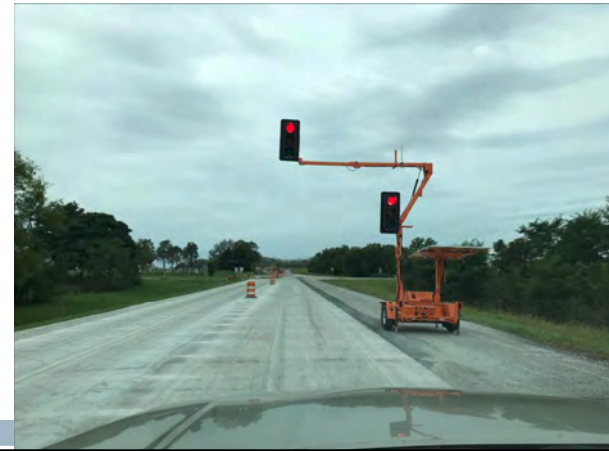
SR 9 - Used Portable Traffic Signals & Pilot Car - on South End of Project
