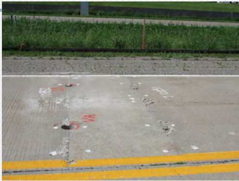
Cell 38, CoVex plate dowels in repair. 5 dowels unsuccessful. Failed in exist PCC
