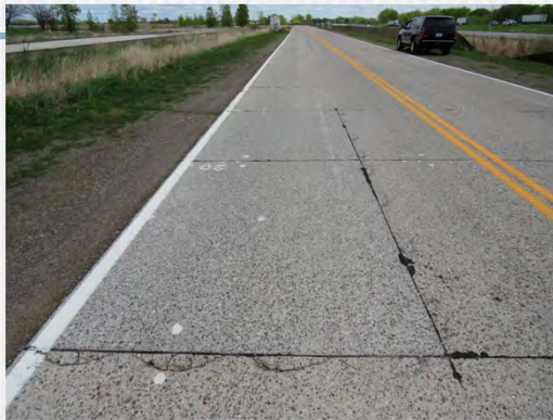
Cell 32, CoVex plate dowels (note failure in original panel, not repair)
