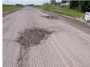
Excessive milling of existing asphalt beyond asphalt lifts (tack line)
