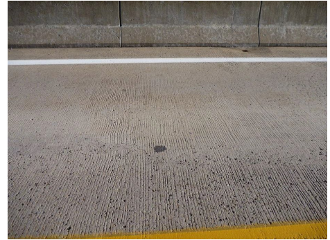
LWC bridged deck on Route 29 after 34 years
