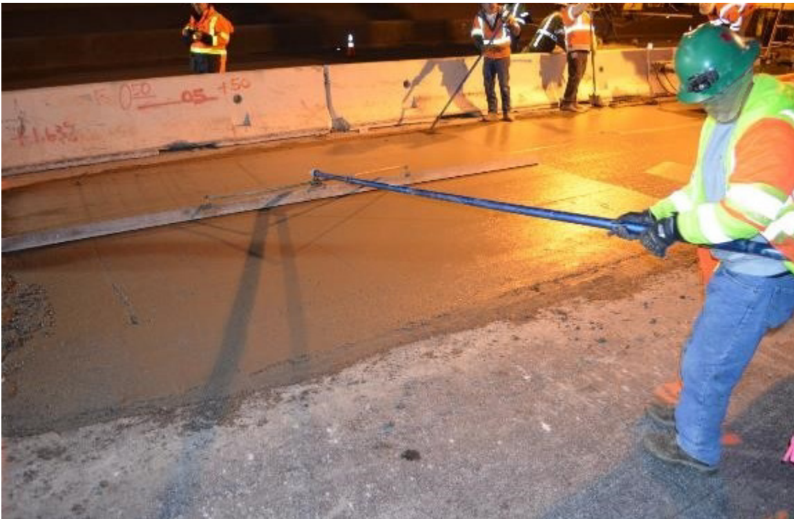
© Applied Pavement Technology
