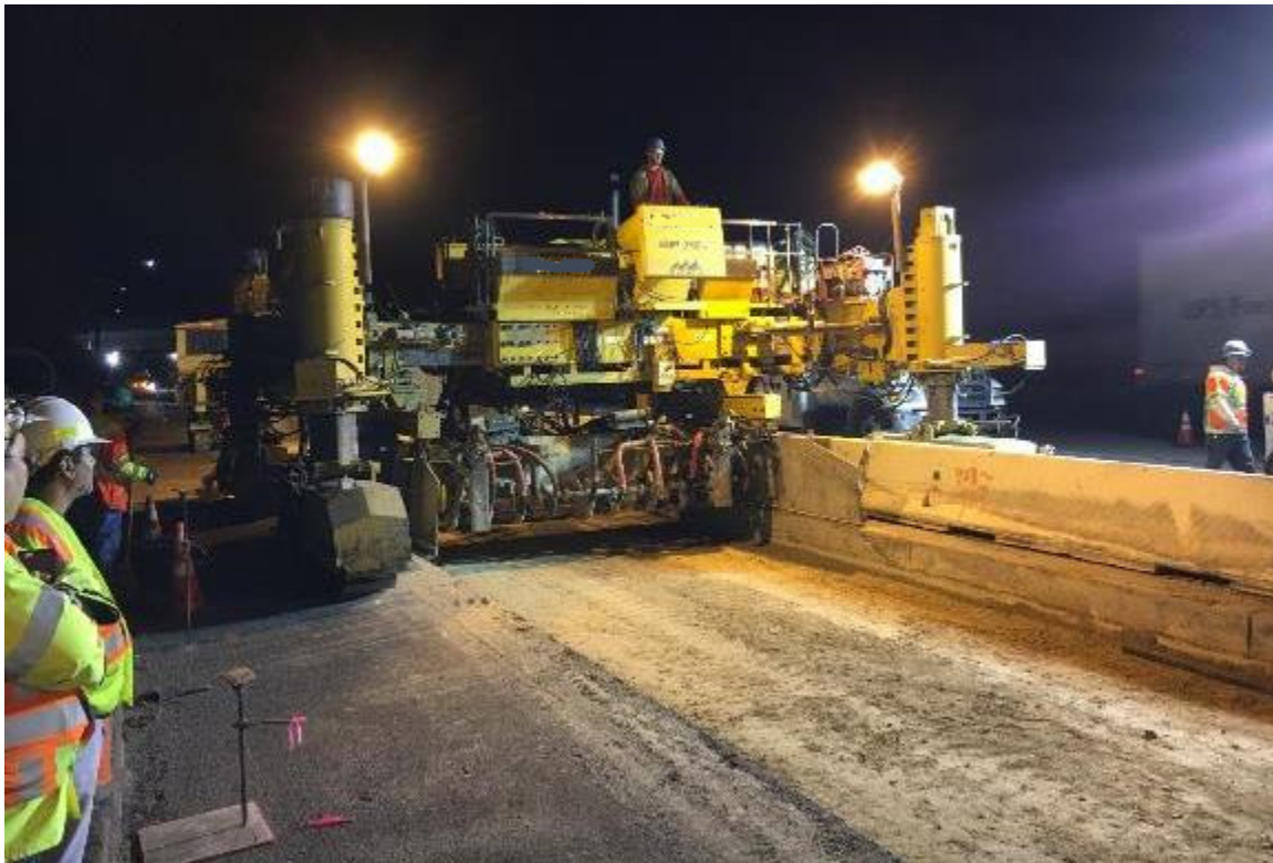
© Applied Pavement Technology
