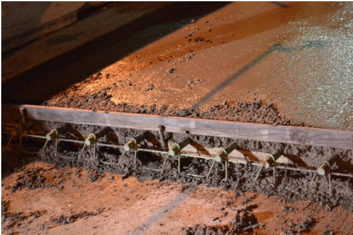
© Applied Pavement Technology
