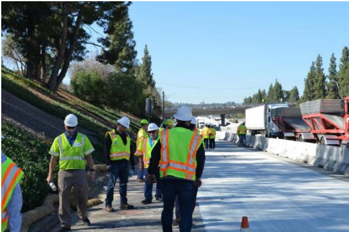
© Applied Pavement Technology
