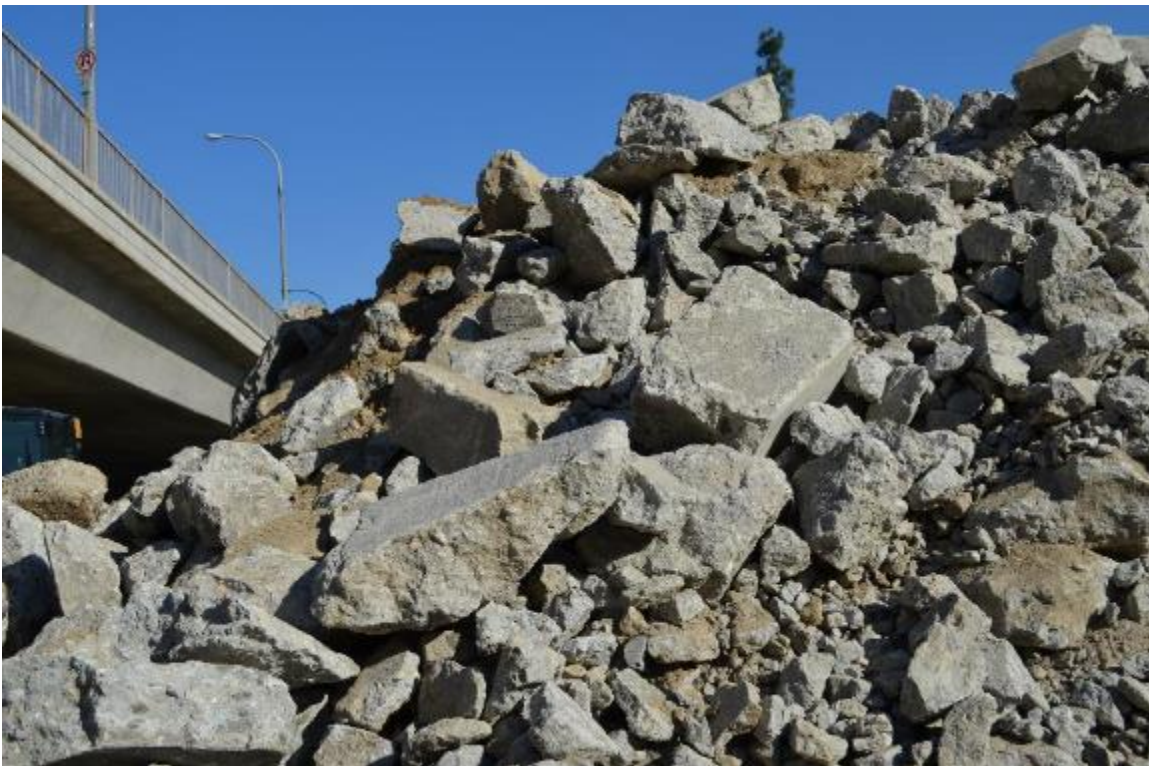
© Applied Pavement Technology
