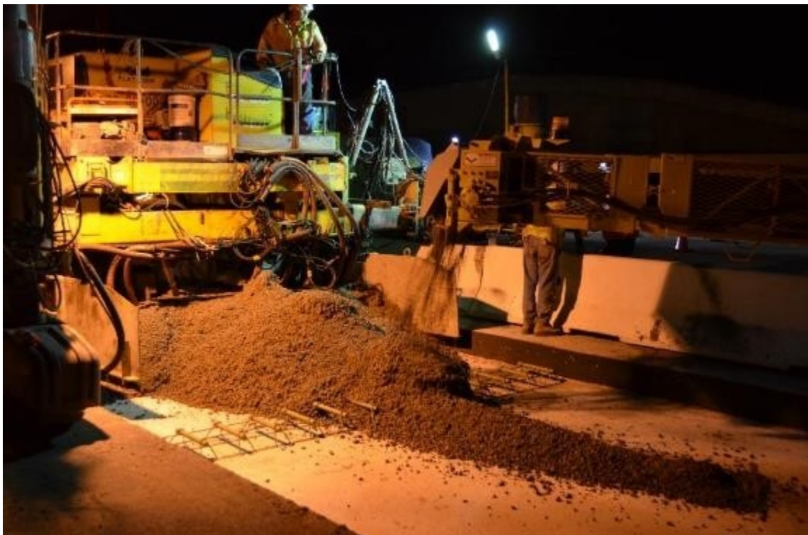
© Applied Pavement Technology
