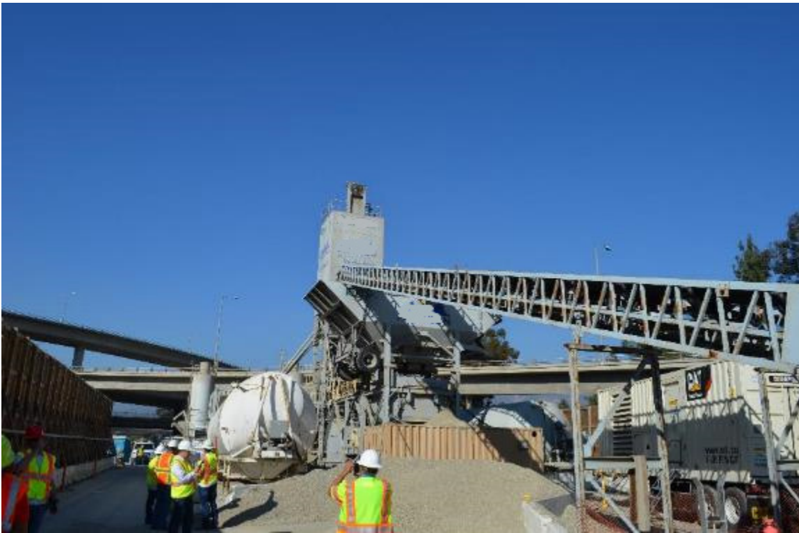
© Applied Pavement Technology
