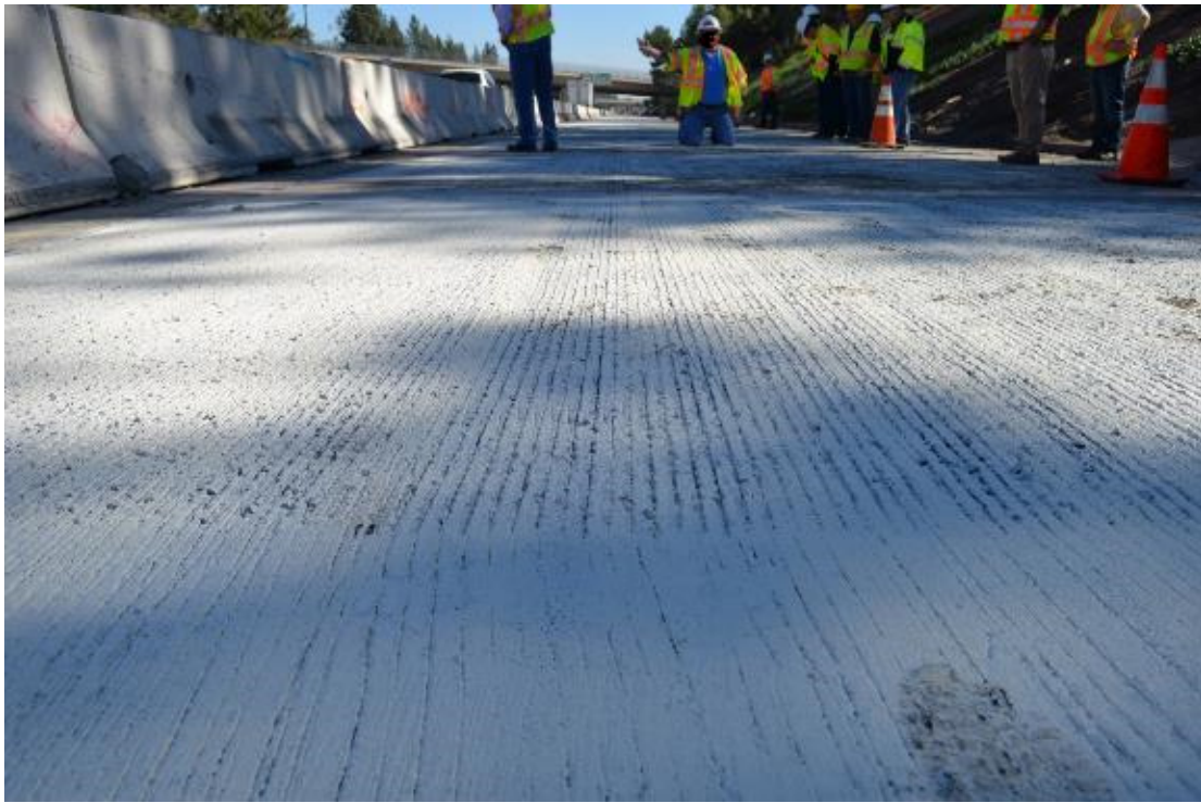
© Applied Pavement Technology
