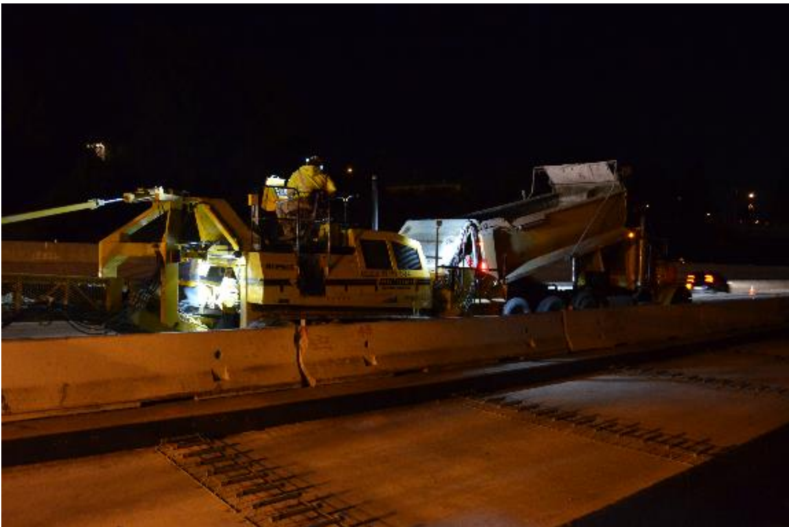
© Applied Pavement Technology
