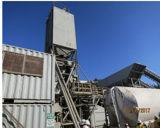
© 2017 Applied Pavement Technology
