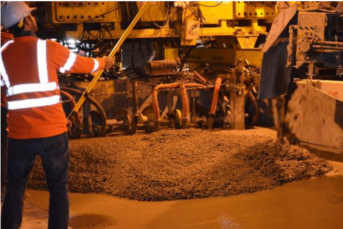
© Applied Pavement Technology
