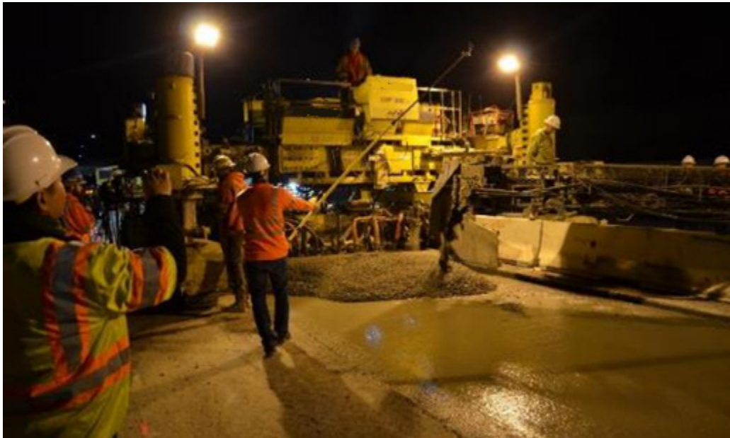
© Applied Pavement Technology
