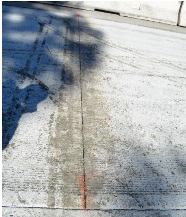
© Applied Pavement Technology
