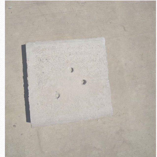
Three holes where concrete powder was extracted
