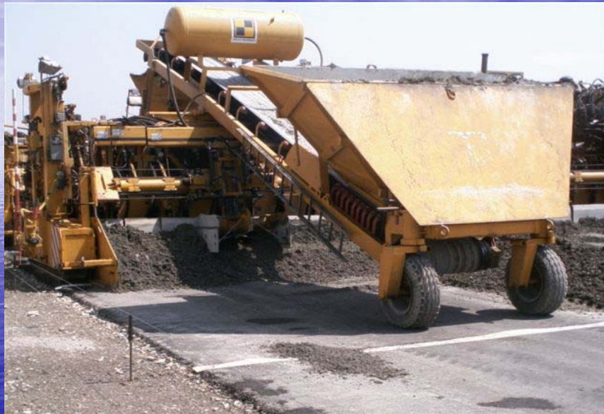
Container for top lift, flat drain in front
