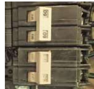
Circuit breaker 60A for each slab
