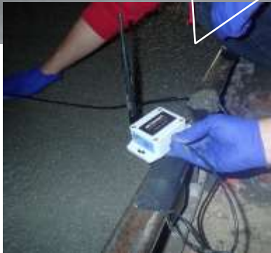
Two wireless humidity sensors
