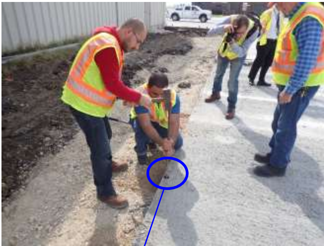
Holes to house wires for sensors system and electrodes
