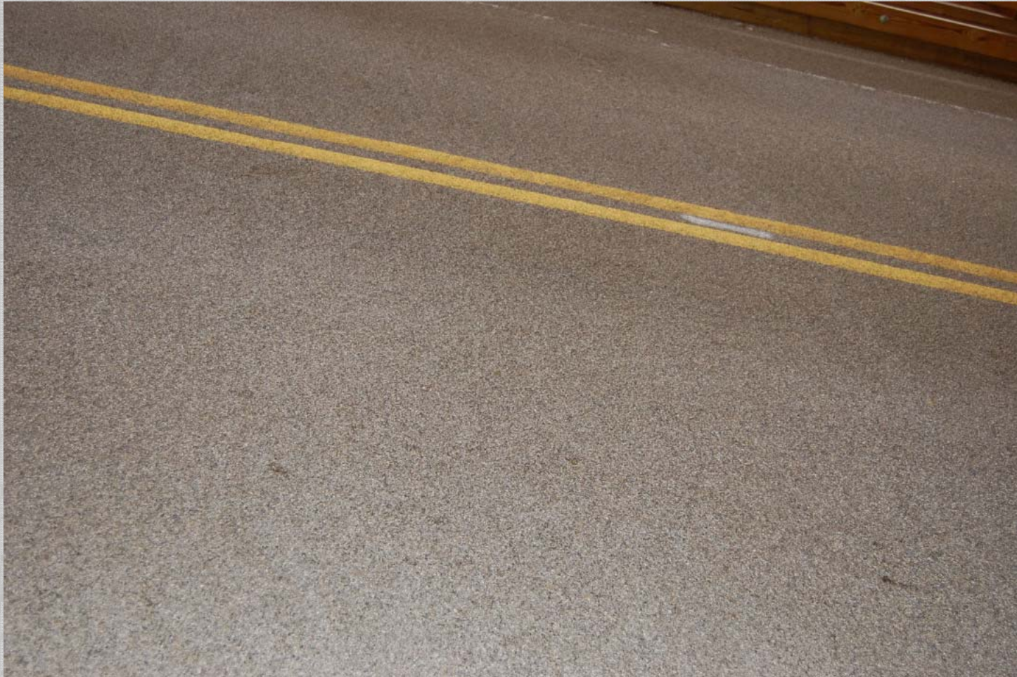
EPOXY WEARING SURFACE
