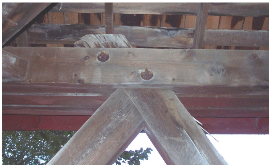
Figure 3. Cataract Bridge. Owen Co, IN (detail). Typical Smith truss post/brace butted joint. Photo: J.A. Barker Engineering
