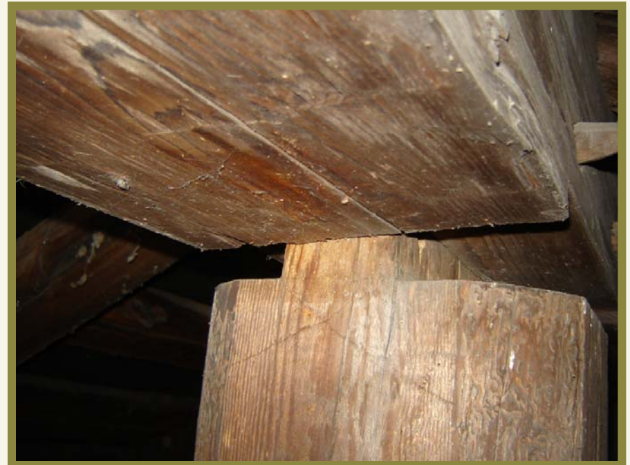
Broken Tenon – Truss Vertical
