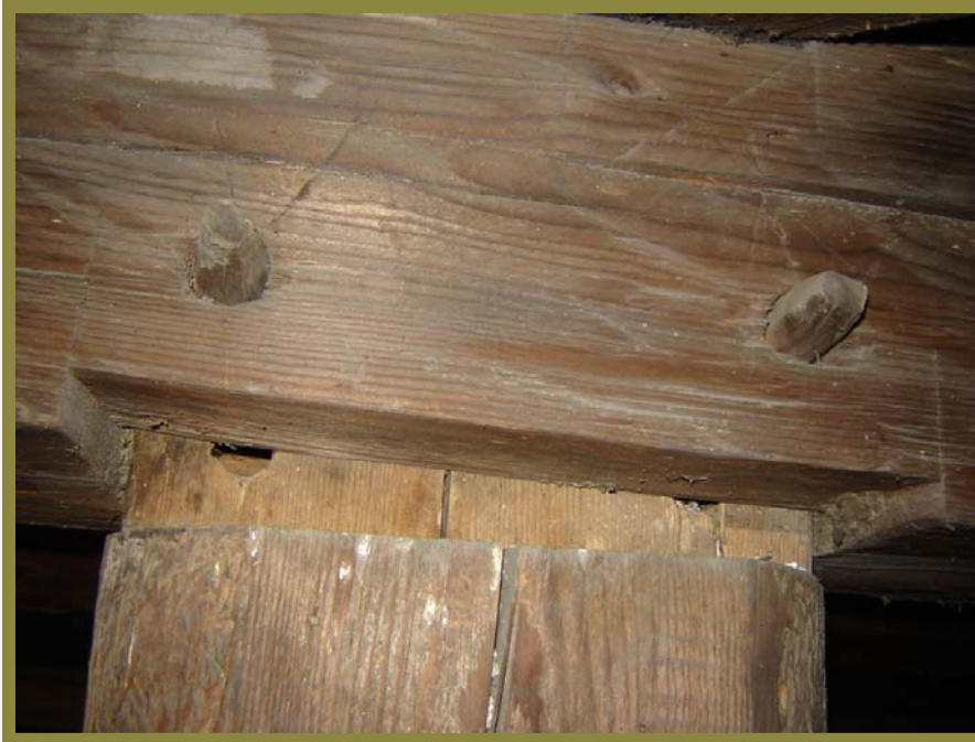
Broken Tenon – Truss Vertical
