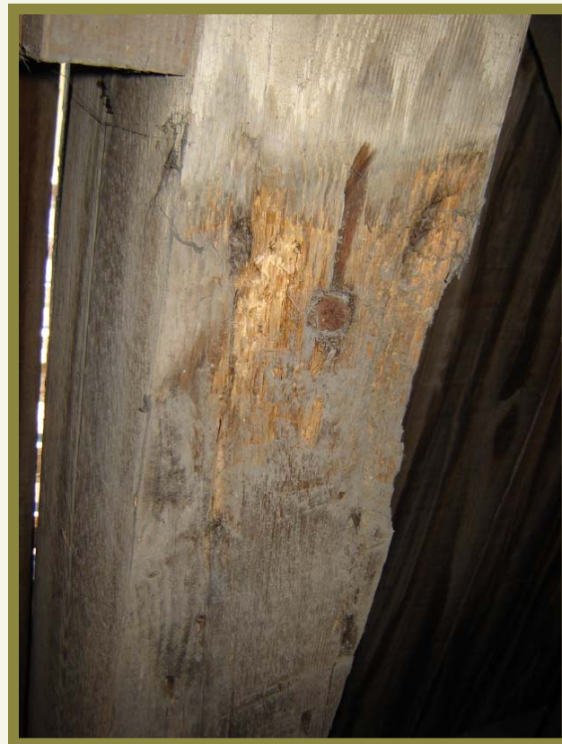
Member Impact Damage
