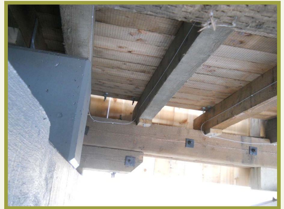
Fire Detection Wires Underside of Bridge
