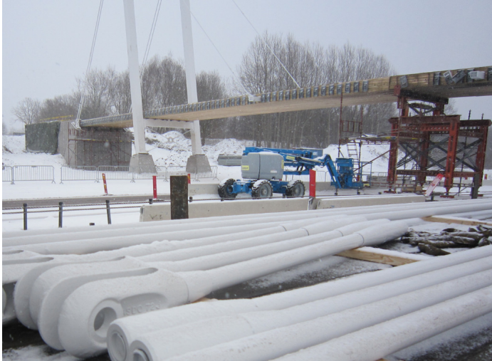
Fig. 17 A detailed procedure was developed for the installation of pylons, deck and stays.
