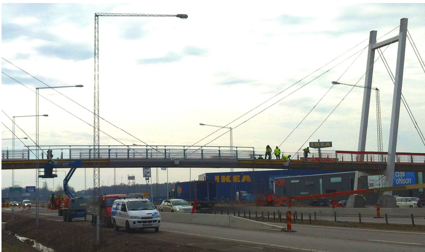
Fig. 19 After installation the bridge deck's sides were covered with thin steel plates
