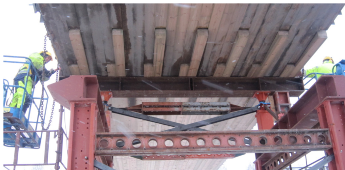
Fig. 16 The prefabricated elements are joined in a 3,0 m long connection zone. Not more than one butt joint occurs in any four adjacent laminations
