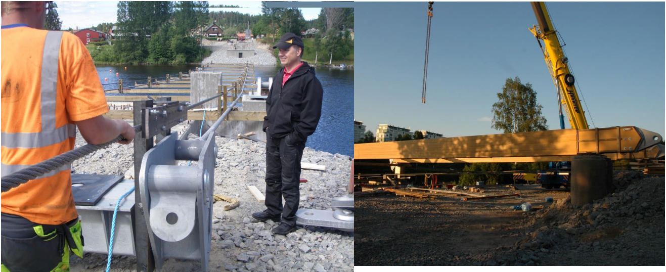
Fig 12: Long bars on their way out (left picture) and assembling of pylon.
