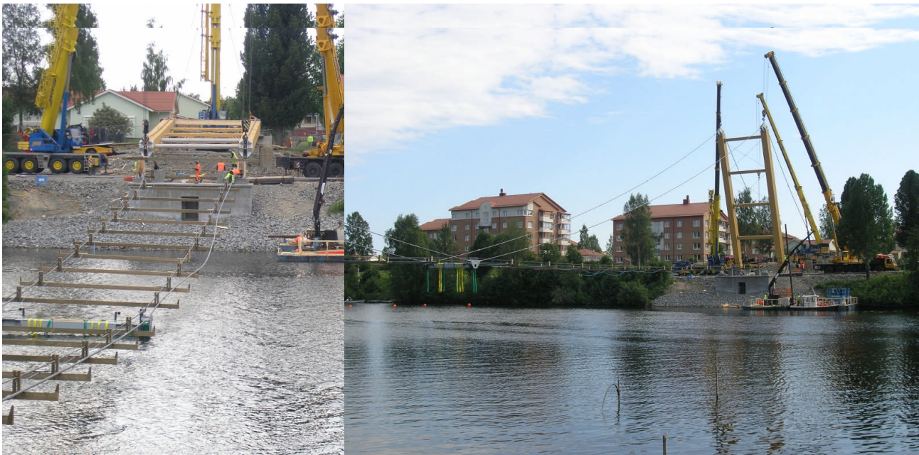
Fig 13: Start lifting pylon (left picture) and pylons almost in final position (right picture)
