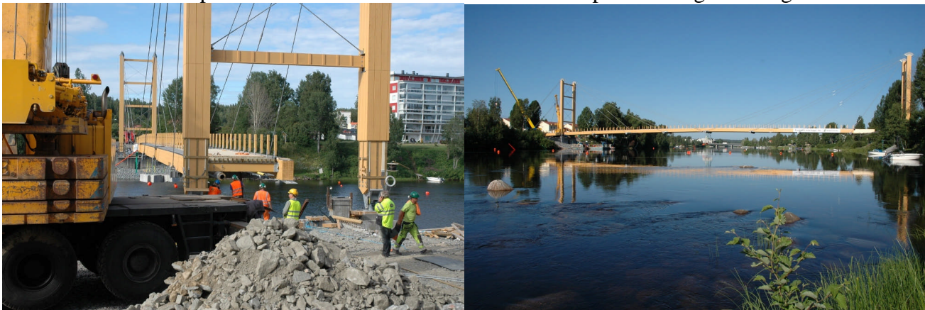
Fig. 14: Bridge on its way out in left picture and almost in final position in right picture.
