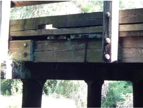
Fig. 12 View of deteriorated wood deck
