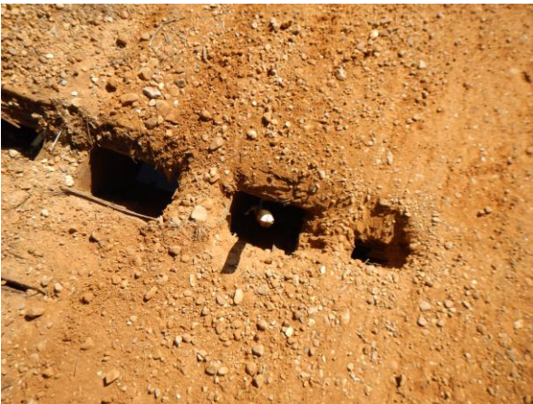
Fig. 18 Loss of deck section spanning stringers
