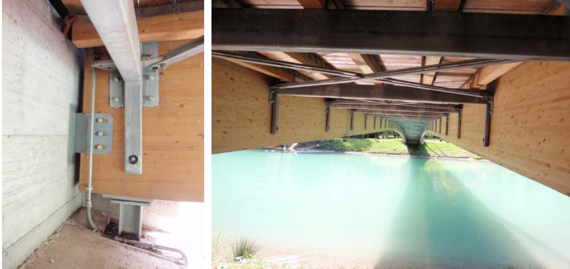
Fig. 3 A detail of the beam support (left). View of the deck from below: one can see the linking steel transversal beams and the steel braces (right).
