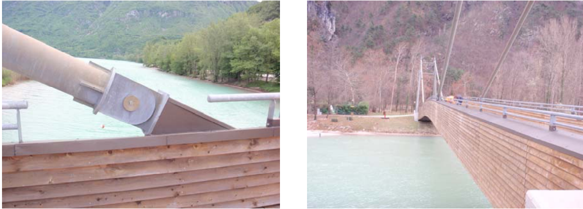
Fig. 5. View of the upper protection system of the beam made by copper (left). A detail of the external larch cladding (right).
