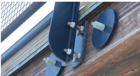
Fig. 5 Parapet post which do not lead water to the deck
