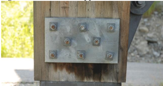
Fig. 8 Exterior steel plate collects moisture.
