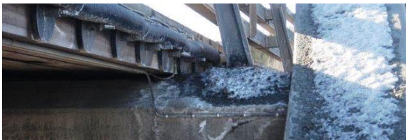
Fig. 15 Dirt on the cross-beam
