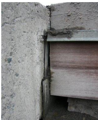
Fig. 10 Open abutment shelf which collects water, dirt and gives high moisture to the sill
