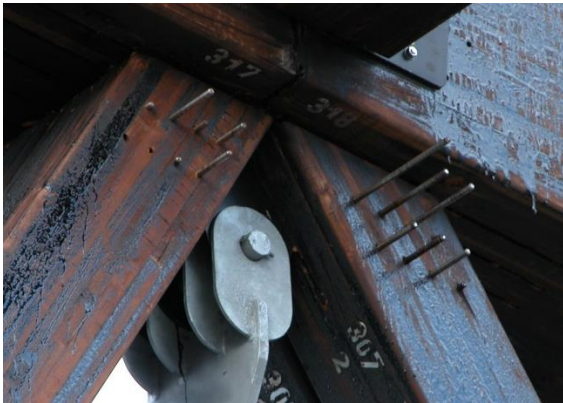
Fig. 19 Dowels dislodging from the structure
