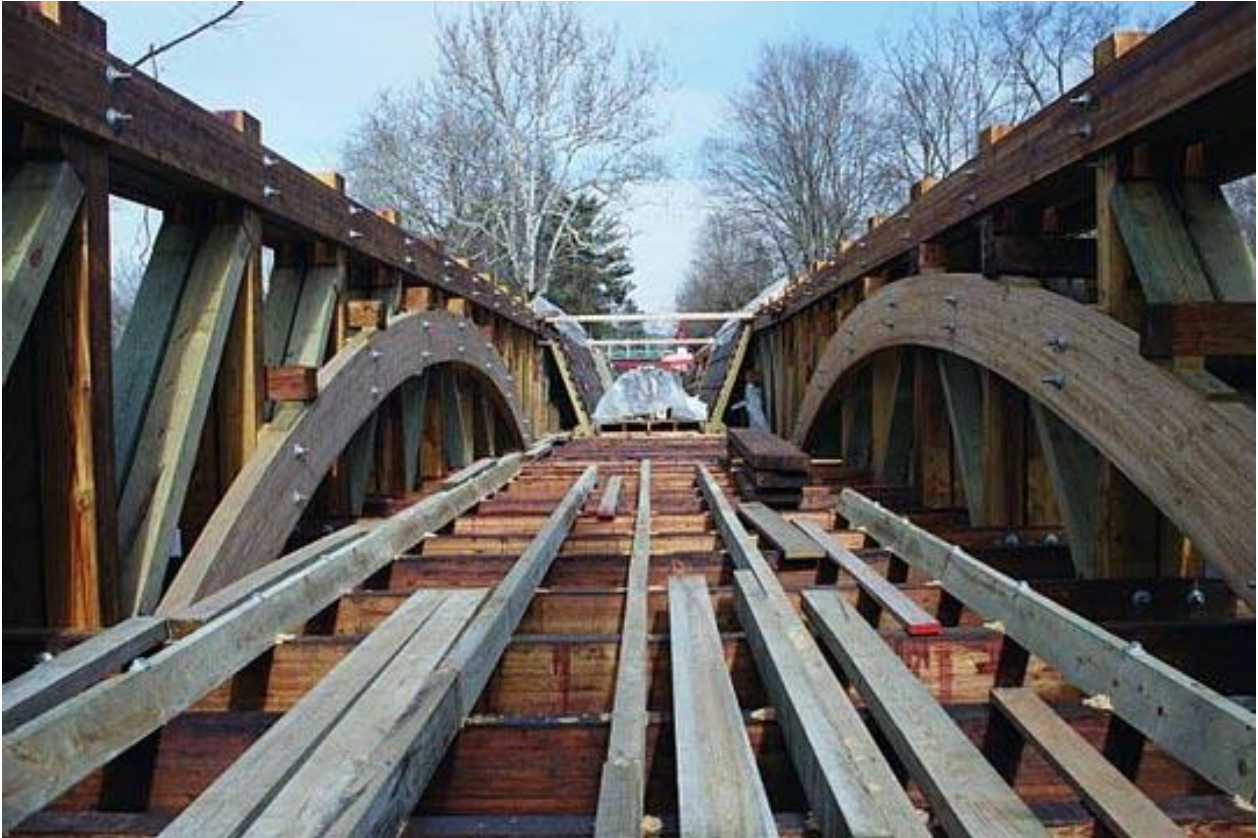
Fig. 7 View to north between trusses with transverse beams in place and trunk framing under construction
