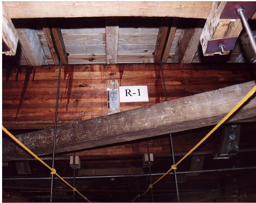
Fig. 8 Field instrumentation on the Aqueduct (rods and rope are the catwalk system)
