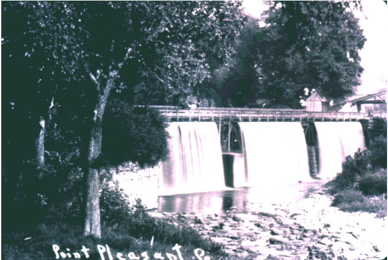
Fig. 3 The western elevation of the steel truss version of the Tohickon Aqueduct with cascade overflows
