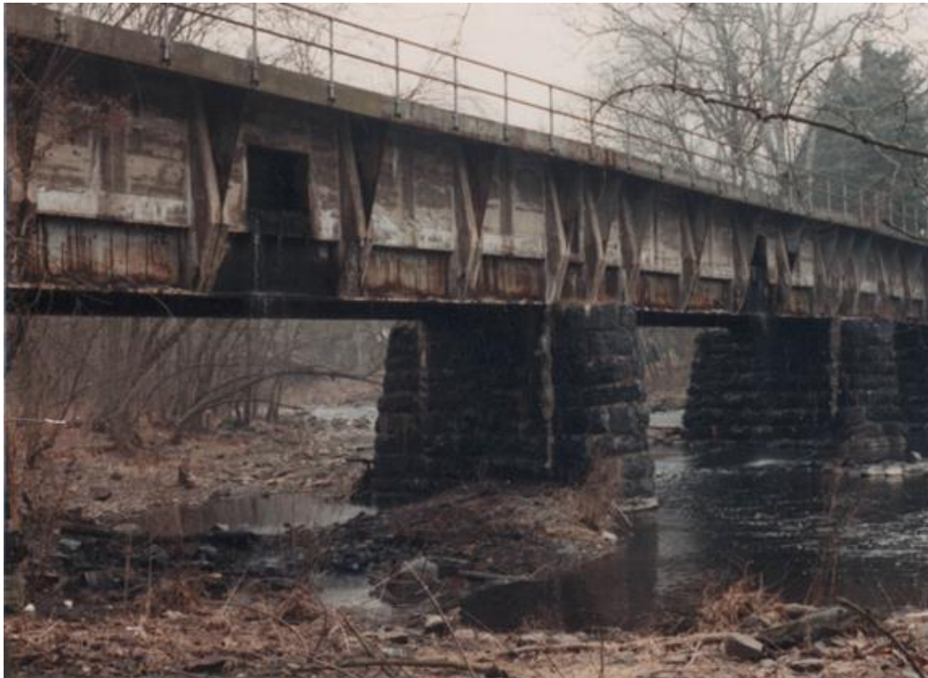
Fig. 2 The previous concrete and steel version of the Tohickon Aqueduct, built after WWII
