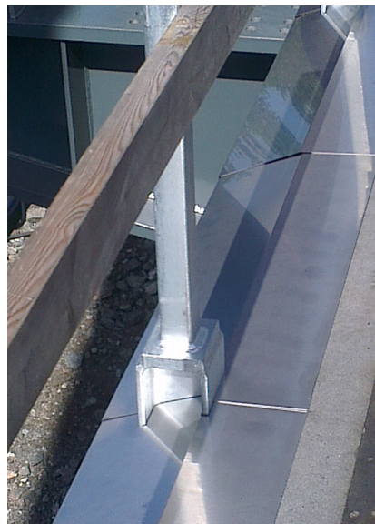
Fig. 8 Bent sheet metal to divert water (before sealing board and asphalt are added)
