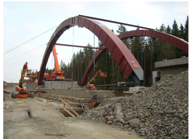
Fig. 12 Both arches in place with temporary support beam. The pontoons are visible to the left in the figure.
