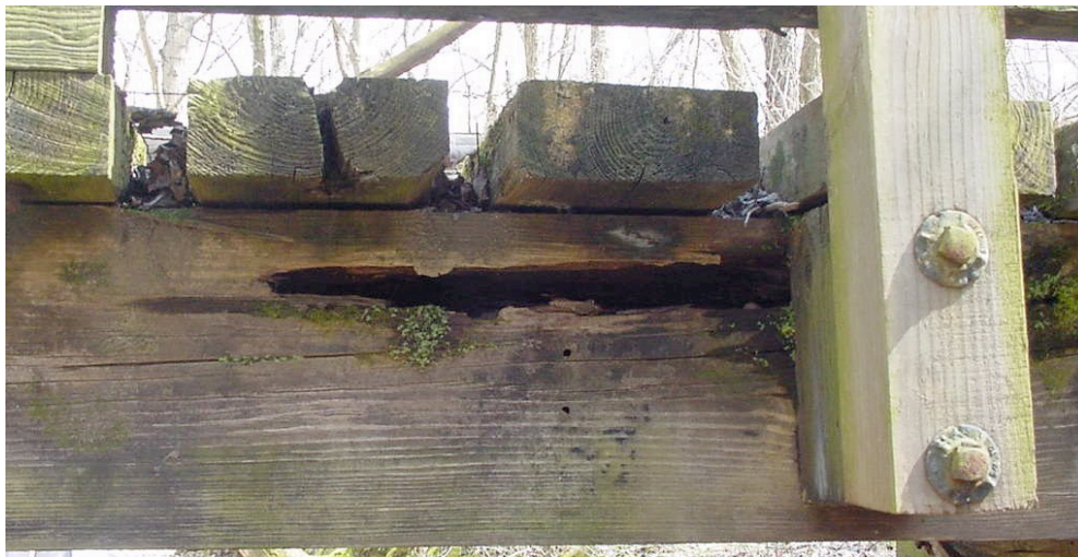
Fig. 2 Hollow section caused by advanced decay
