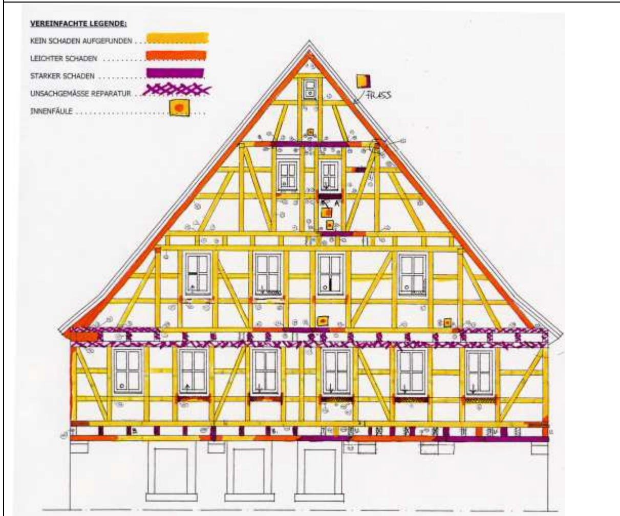
Fig. 5: Overview sketch with a simplified color coded condition inventory. This inspection was carried out by one person on one day including the drawing of the inventory what is usually done on site.
