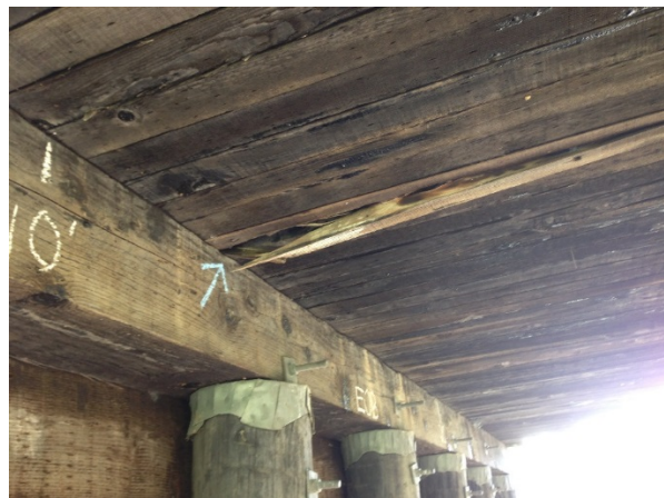
Fig. 13 Damage at longitudinal deck panel connection, Clarke 3
