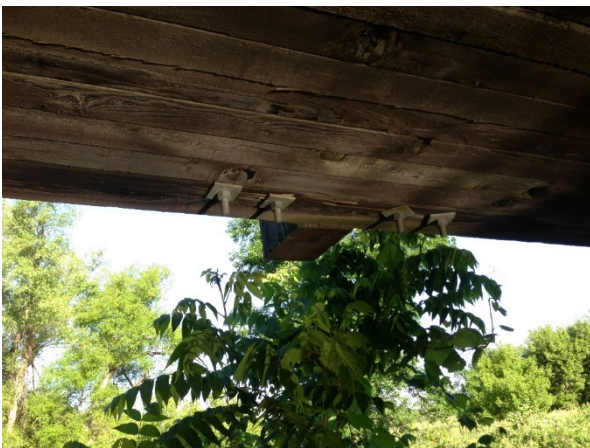
Fig. 12 Damage at connection detail between guardrail post and deck, Clarke 3
