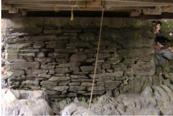
Failing abutment, Green River Covered Bridge, MA.
