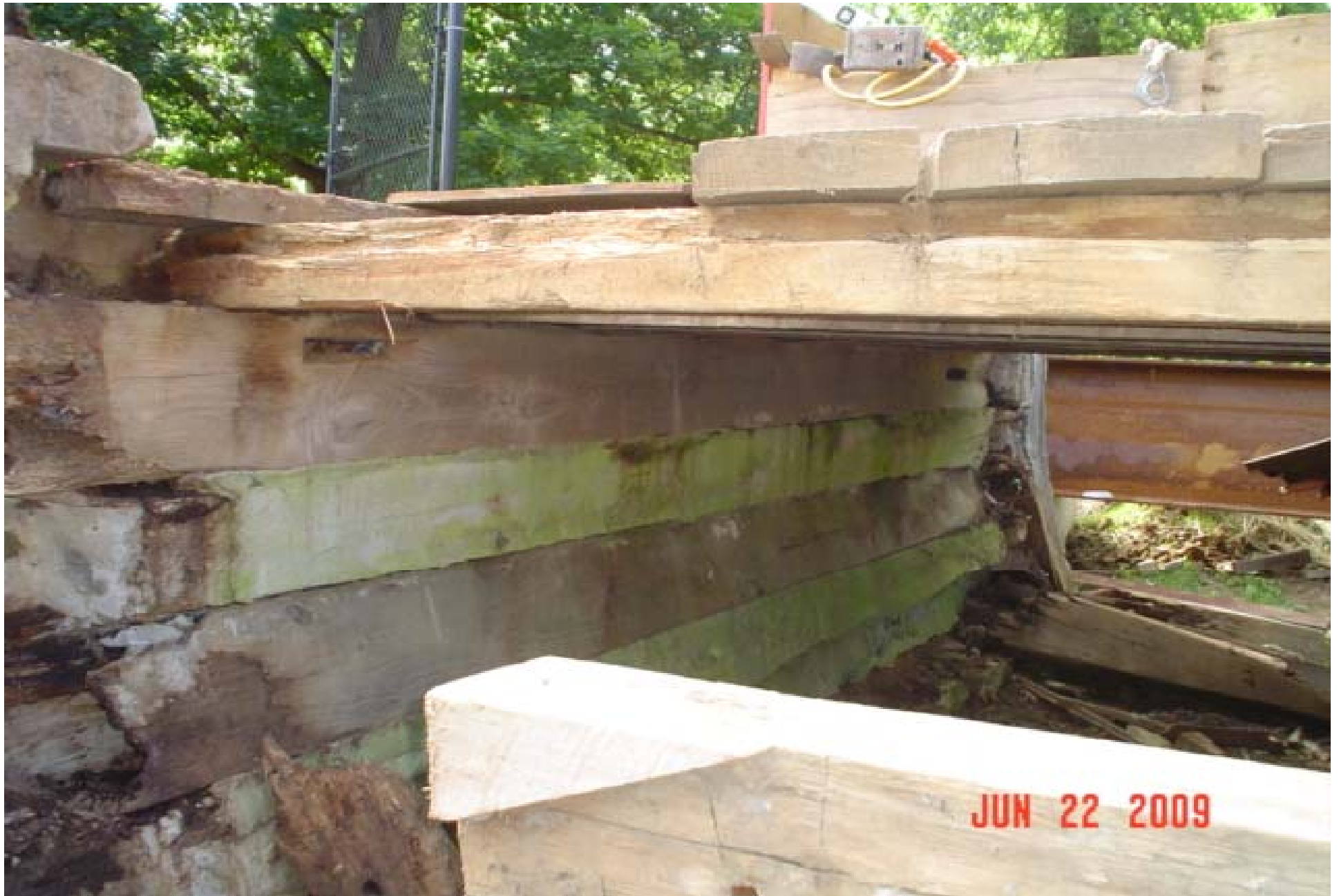
Embedded arch bearing timbers; severe decay at arch contact points
