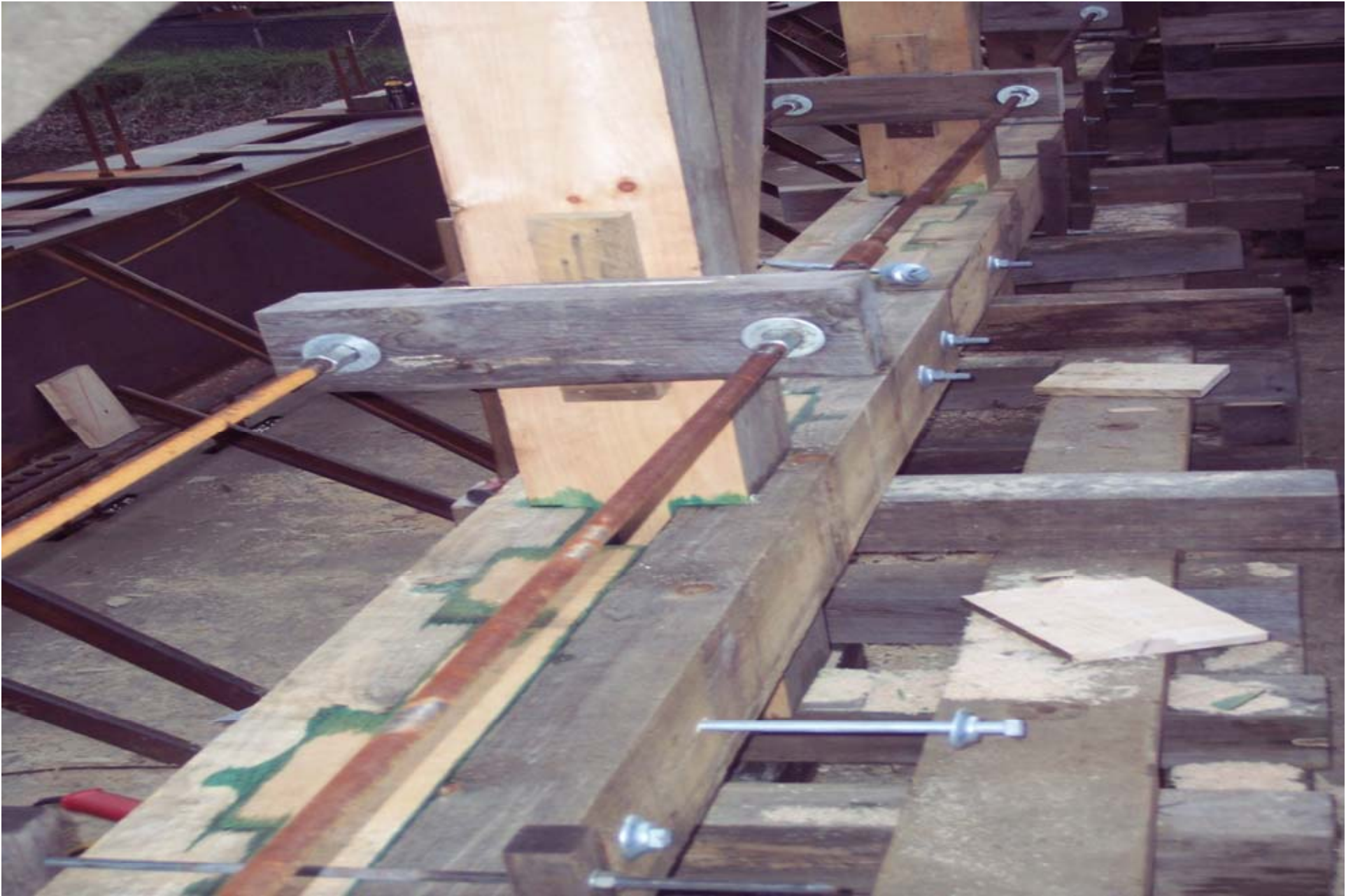
Design change for shear connections- double the inclusion, double the shear “heads”
