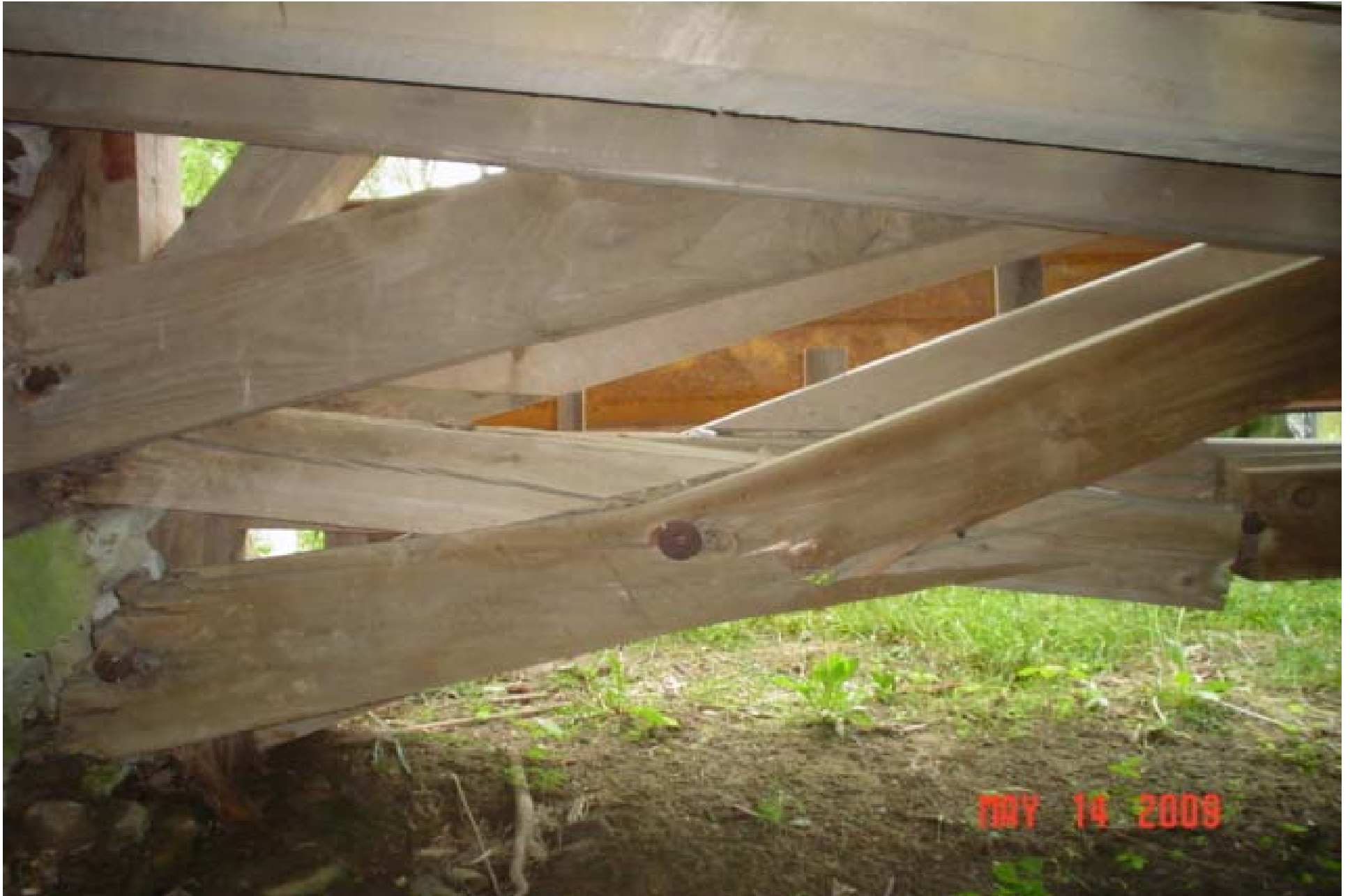
Arch/ bottom chord failure
