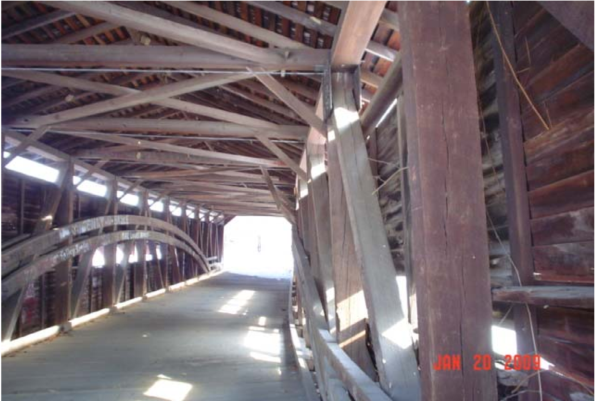
Gilpin's Falls before rehabilitation- lateral bow 18.5", 12.5" sag
