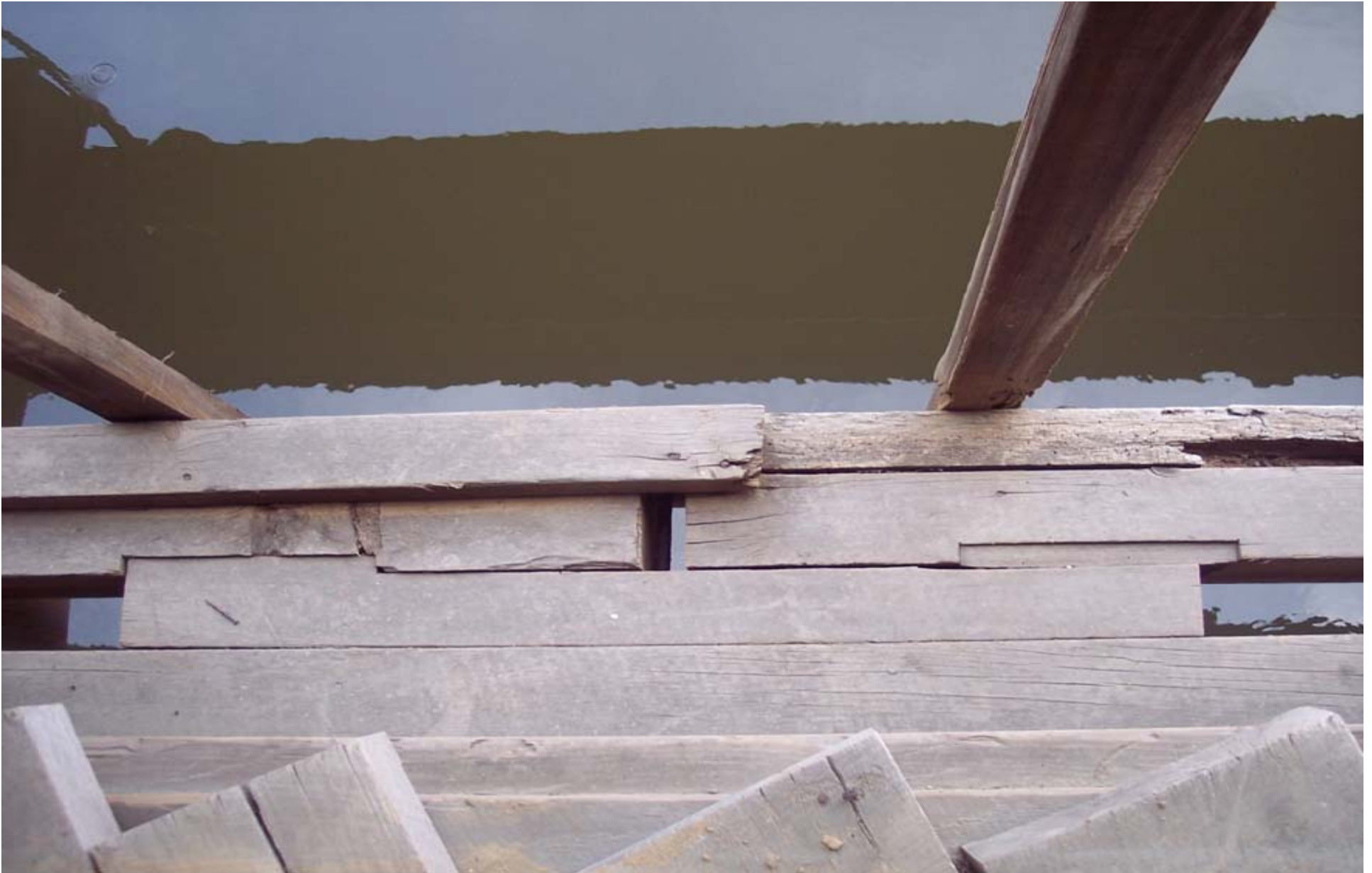
Typical shear key failure
