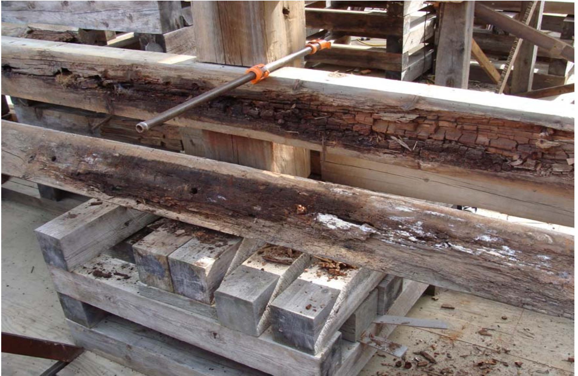
1930's splice plate accelerated decay
