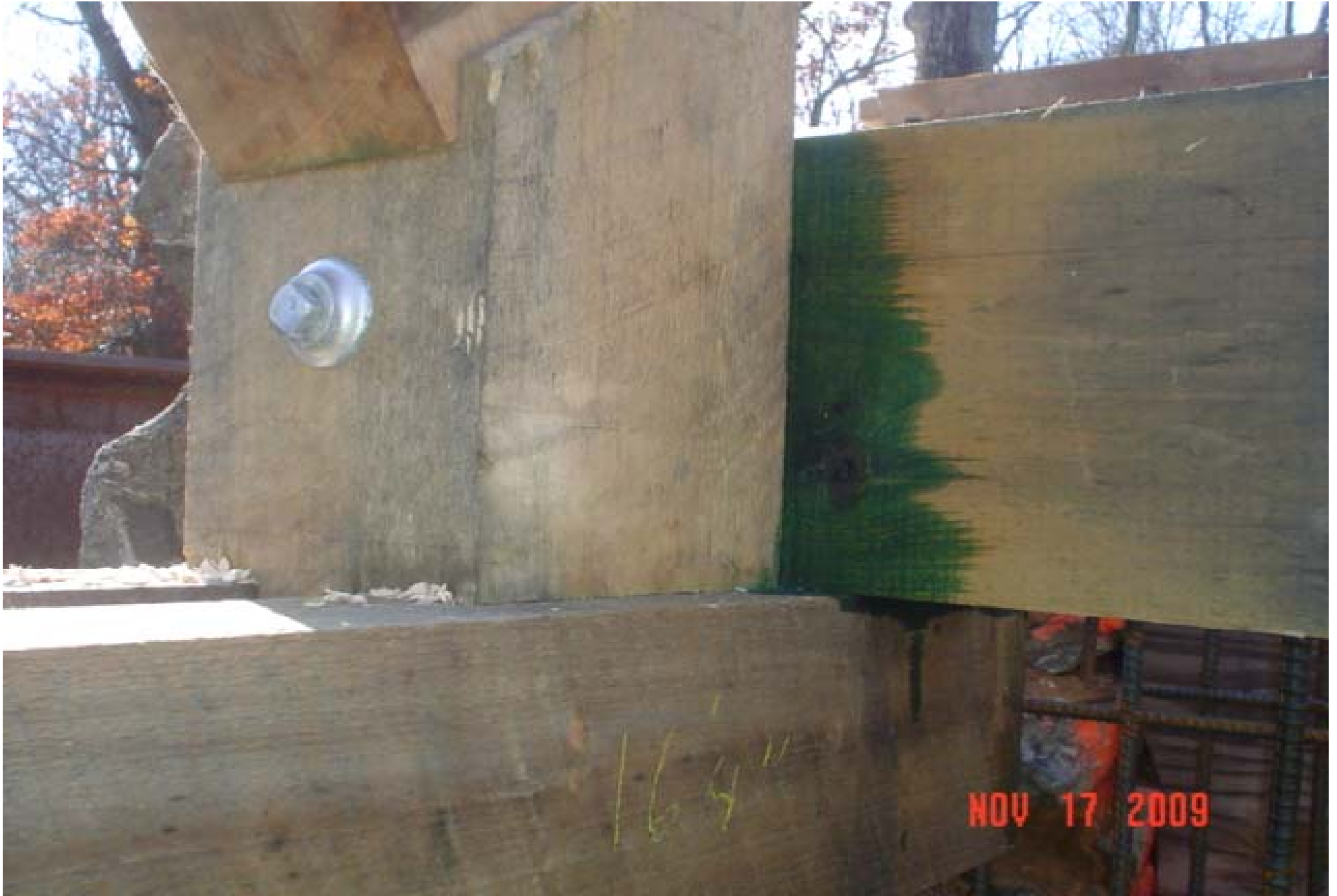
Tight joinery, preservative treatment at member interface, bolt head orientation
