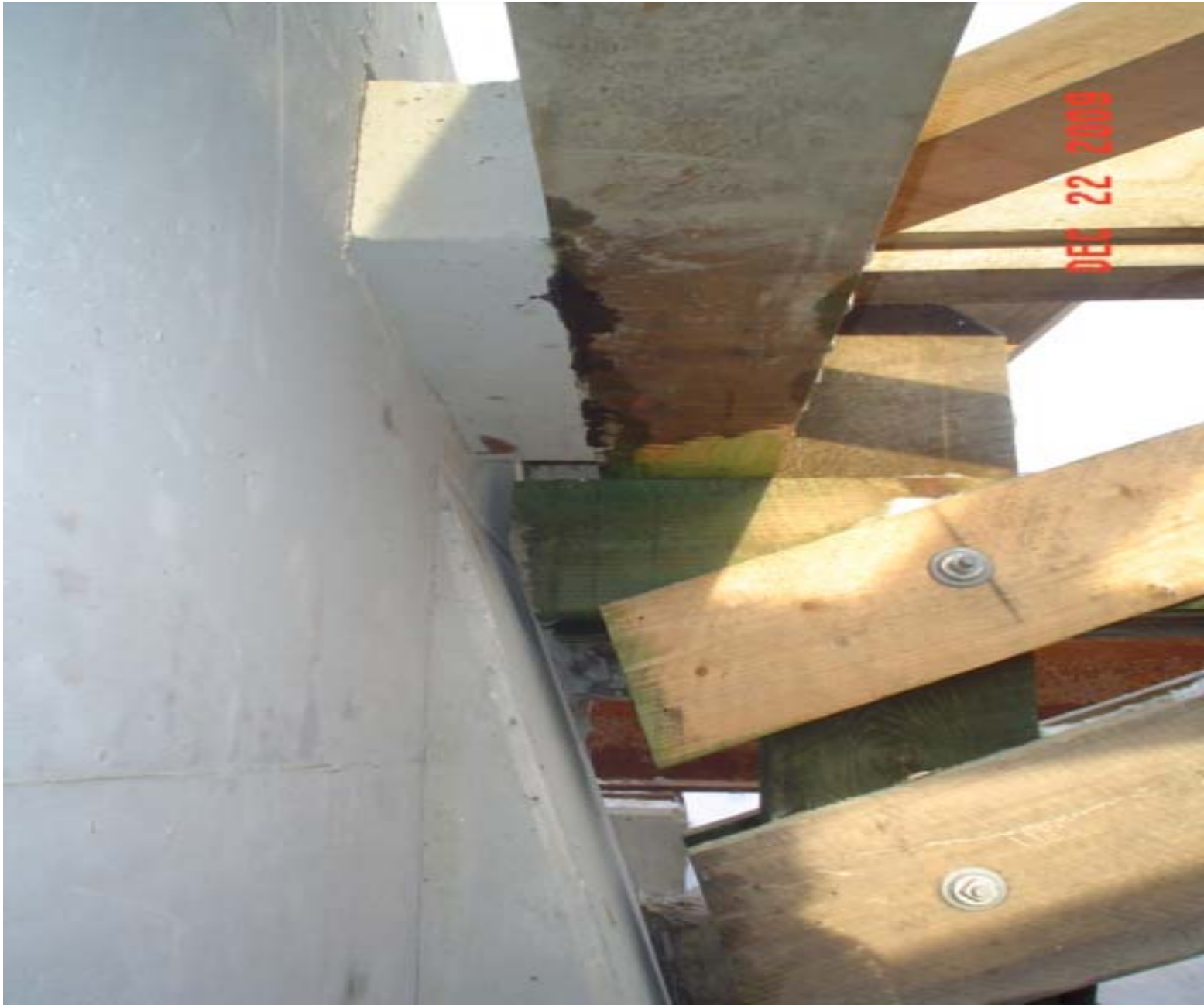
New concrete thrust wall, gaps designed to facilitate free movement of air
