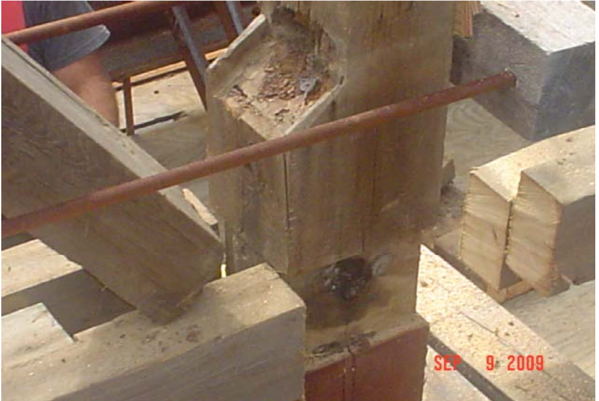
Water fed decay from post/ brace “step” clear through to chord connection
