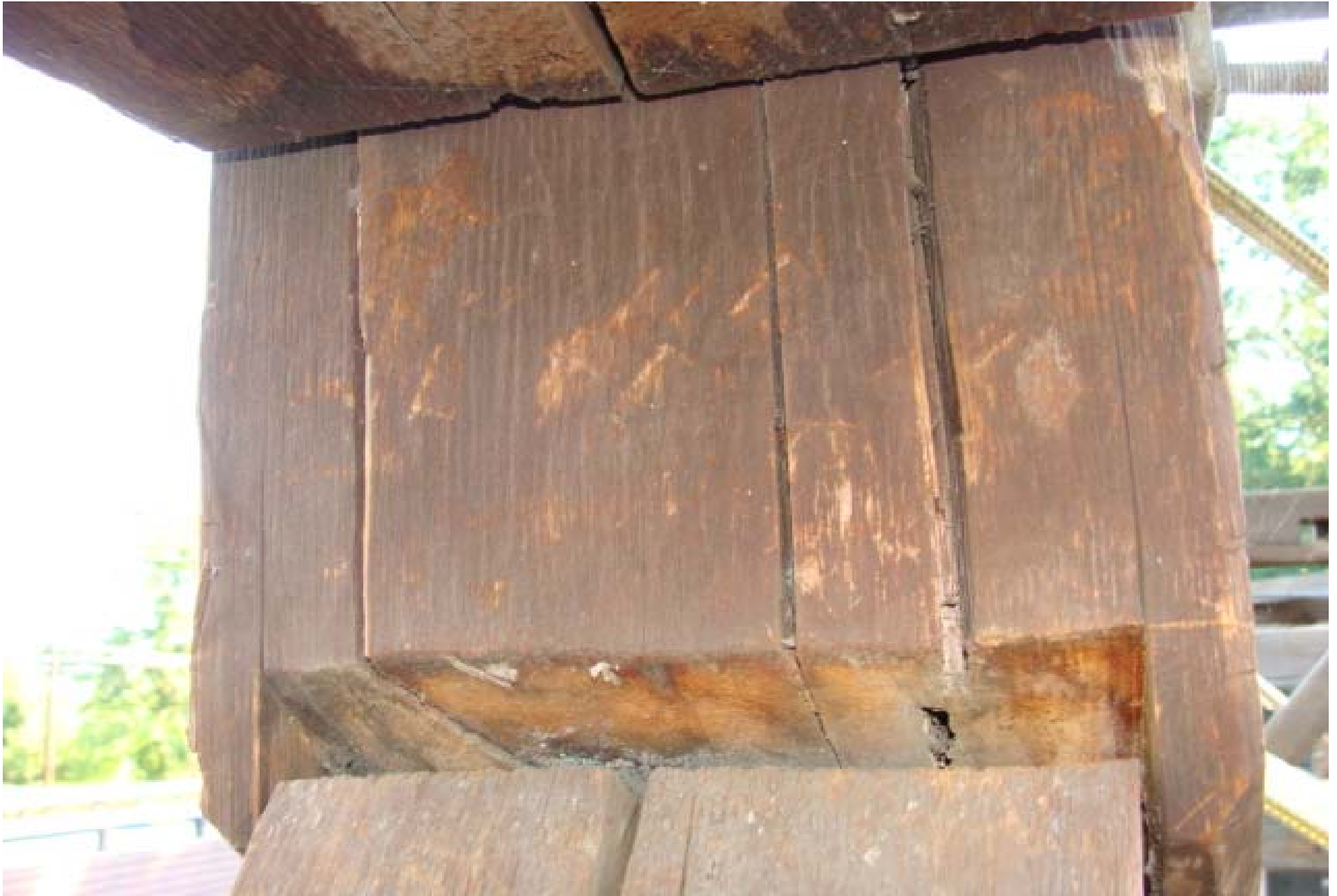
Shear failure post top
