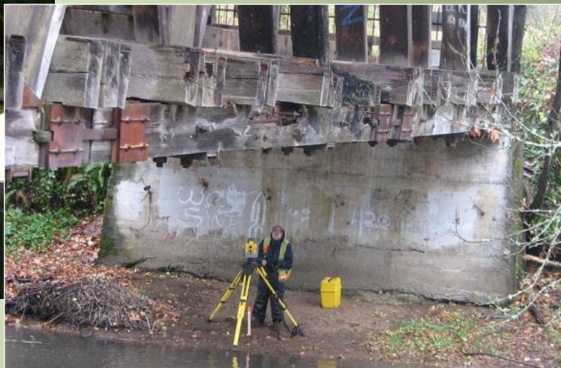
Fire on bottom chord near mid-span
