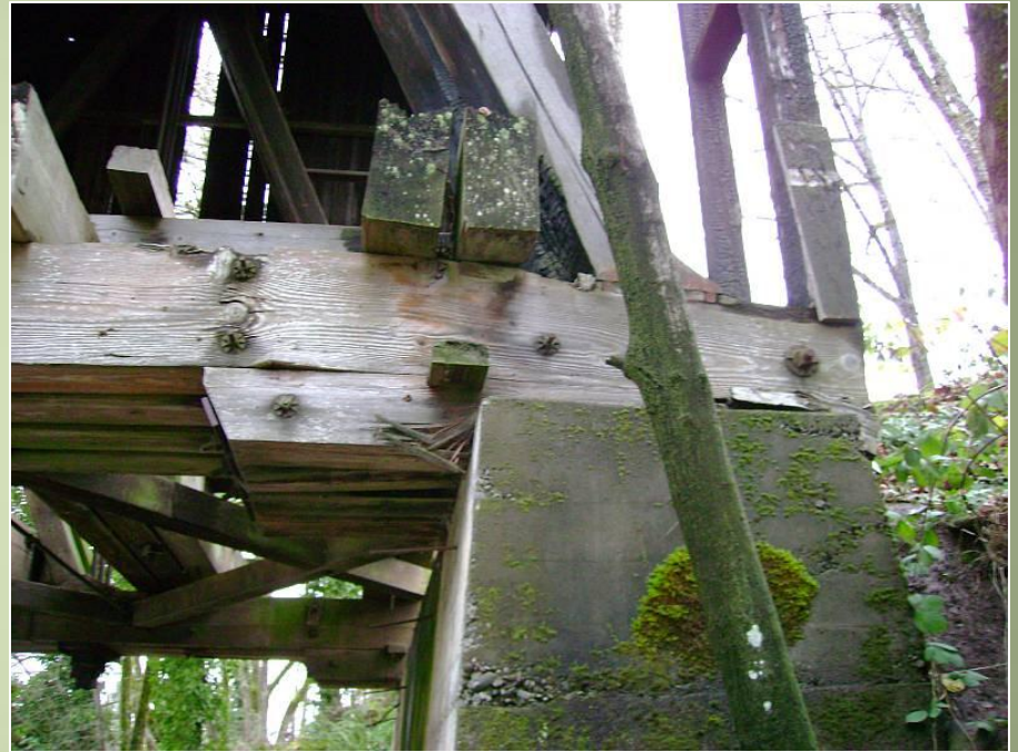
Bottom chord crushing at both ends
