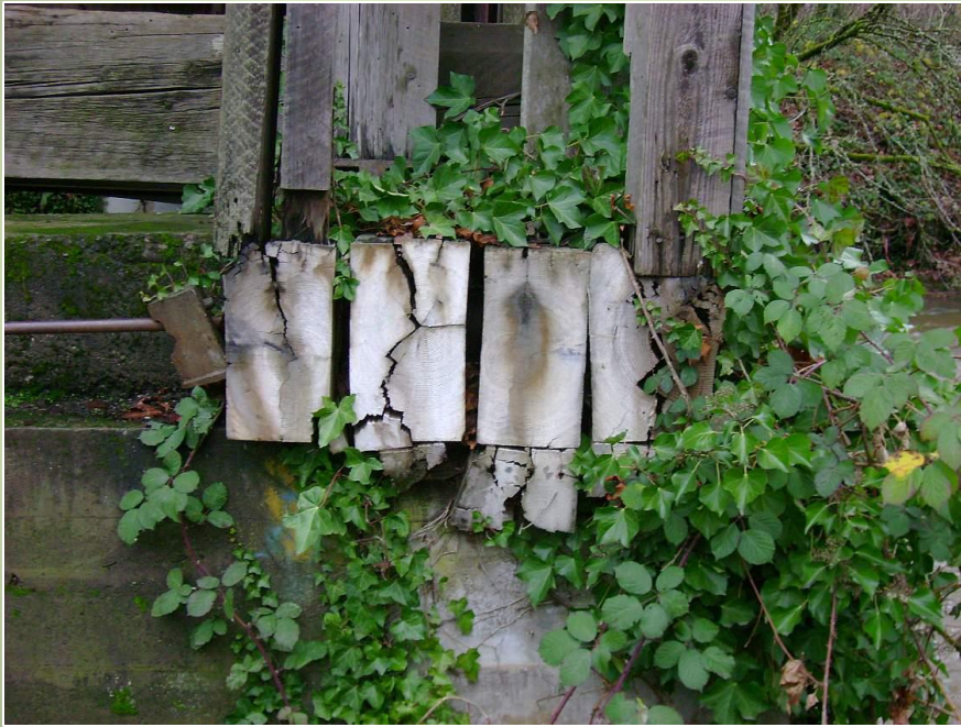
Corbels upstream side rotted away completely
