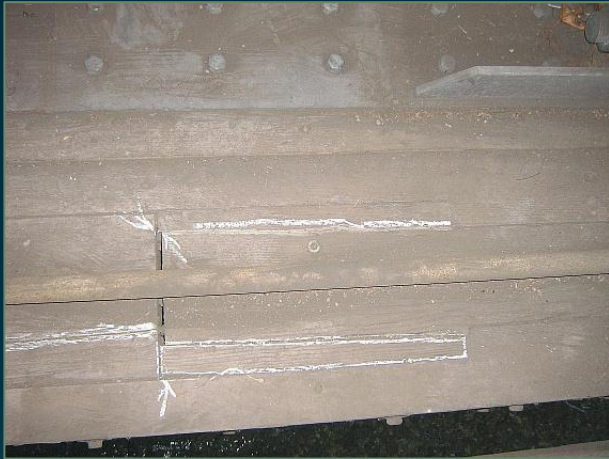
Broken splices leaving gaps to 1/2"
