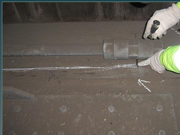
Gaps not closed by tie rods
