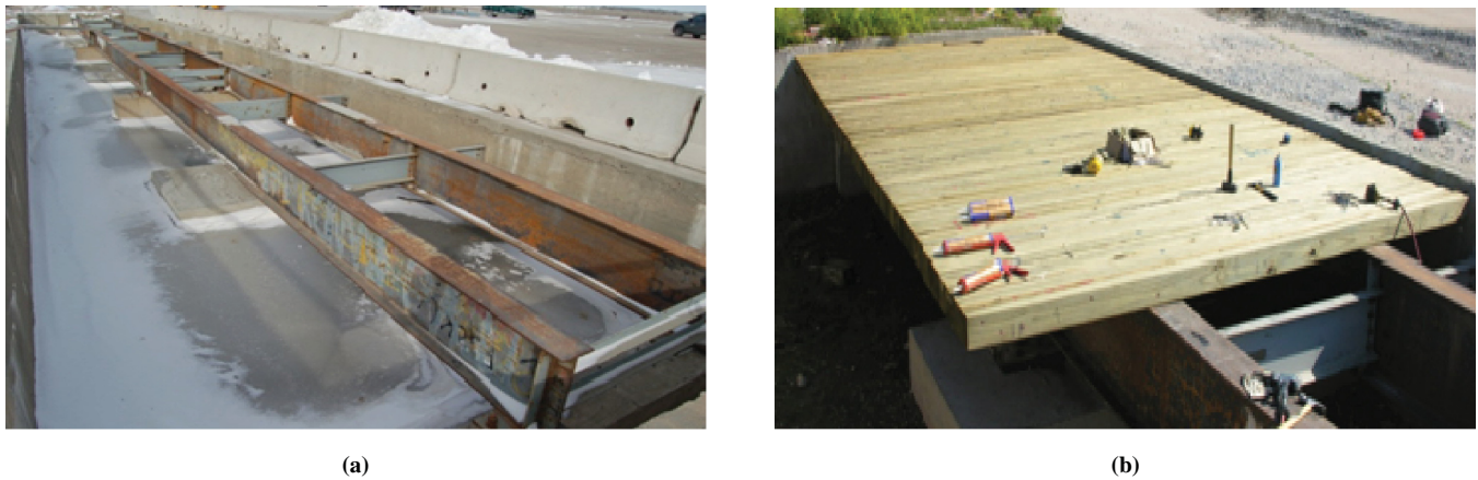
FIGURE 1 Full-scale bridge deck constructed for testing: (a) substructure and (b) details of transverse nail-laminated deck.
