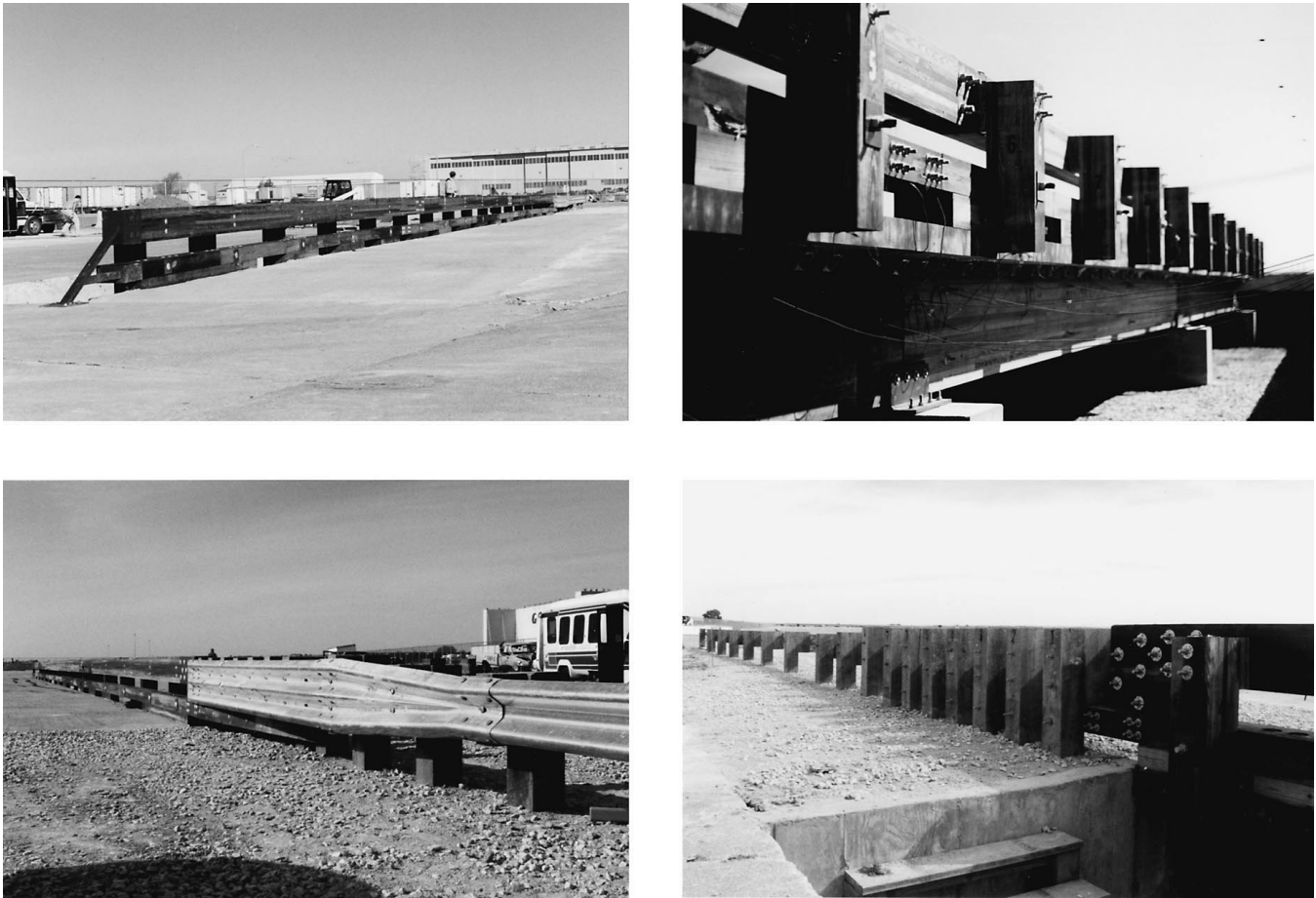
FIGURE 1 System No. 1: glulam rail with curb bridge railing ( top ) and thrie beam with curb transition ( bottom ).
