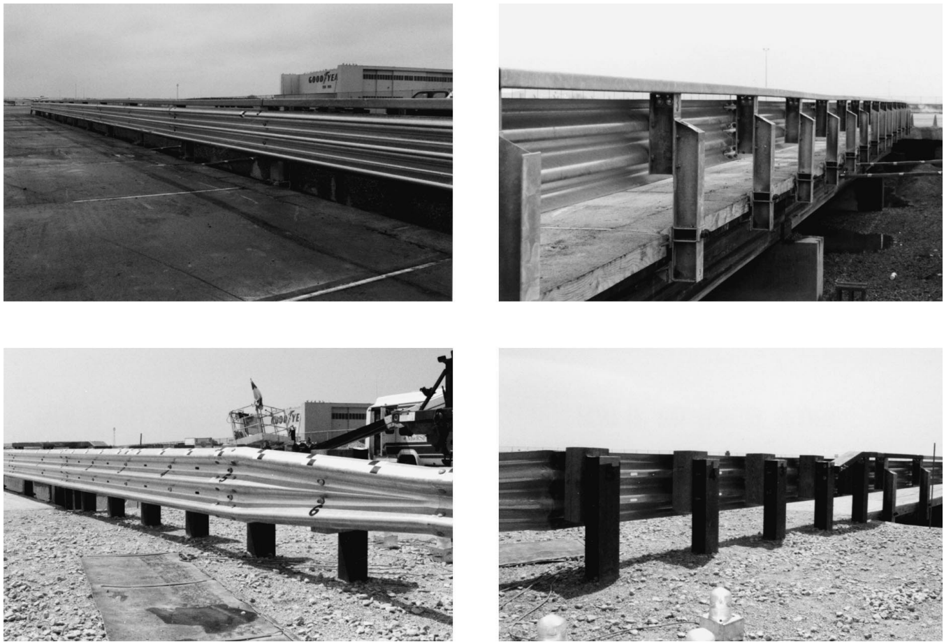
FIGURE 2 System No. 2: steel thrie beam with tube bridge railing ( top ) and thrie beam with tube transition ( bottom ).
