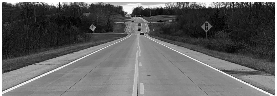
Unbonded concrete overlay on Missouri Route D (Todd LaTorella, ACPA, MO/KS Chapter)
