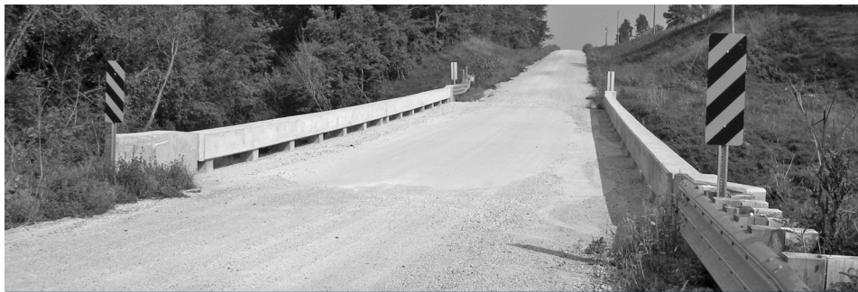
Example of overgrown vegetation at a guard rail
