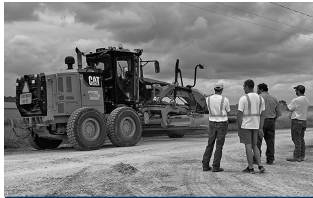
Training attendees view a demonstration of the operation of the equipment
