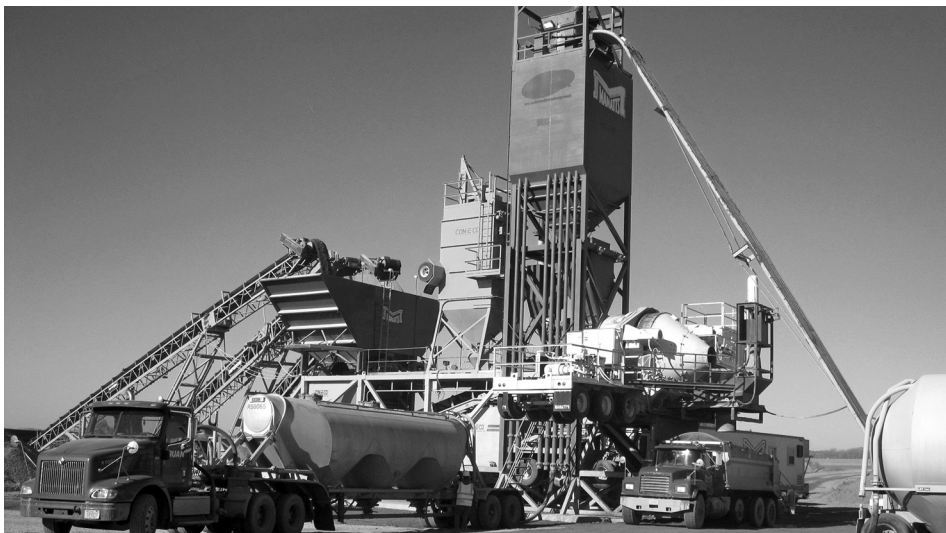
Portable central-mix concrete plant (left and right photos: Jim Grove, ATI Inc./FHWA, used with permission)
