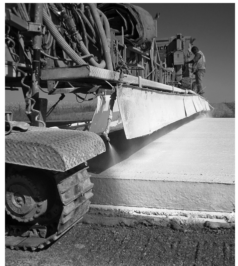
Curing machine coats both the top surface and sides of a slipform paving slab
