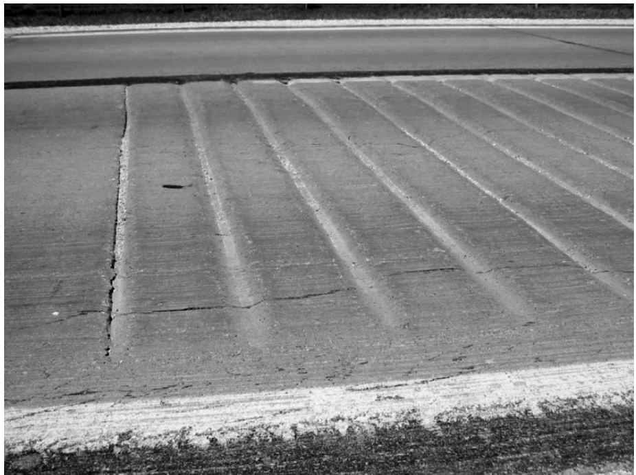
Advance rumble strips on a portland cement concrete pavement. (Photo courtesy of Bob Sperry)
