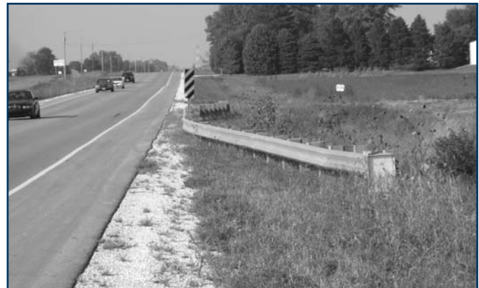
A guardrail around a culvert, protecting from the drop-off hazard. (Photos courtesy of Bob Sperry)
