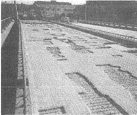
Delamination areas shown prior to placement of Class A repair
