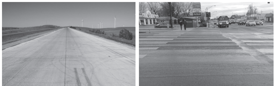
Well done whitetopping of asphalt pavement (left) vs. rutted and otherwise damaged pavement (right).
