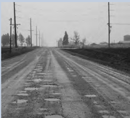
Rural road with potholes and corrugation
