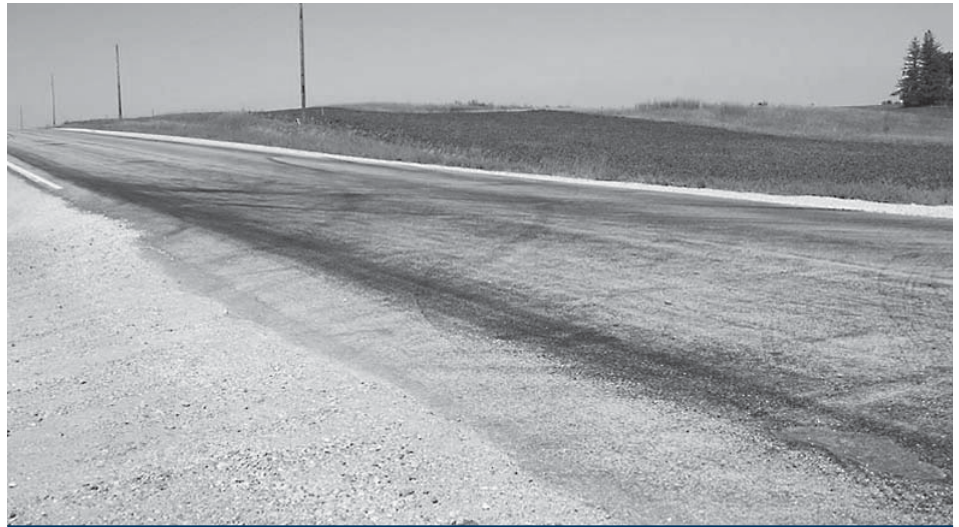
Deteriorating low-volume county roadway in Iowa (photo courtesy of Tom McDonald)
