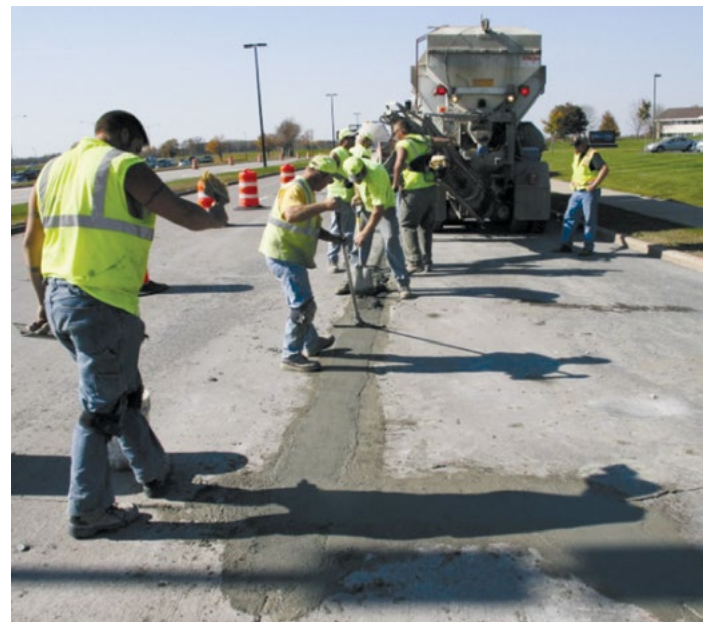
Kevin McMullen, Wisconsin Concrete Pavement Association, from Frentress and Harrington 2012, CP Tech Center
