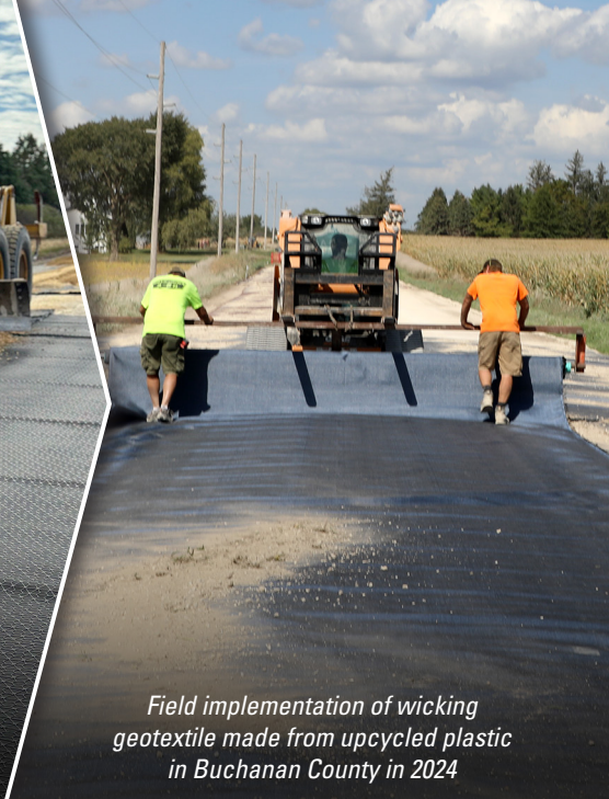
Field implementation of a composite geosynthetic made from upcycled plastic in Buchanan County in 2023
