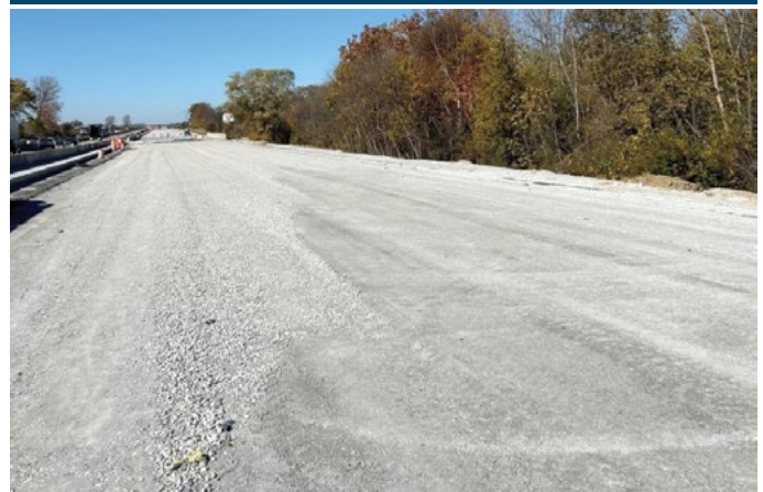
(b) Top of AASHTO 53 subbase on October 27, 2024, looking west from the east end of the project
