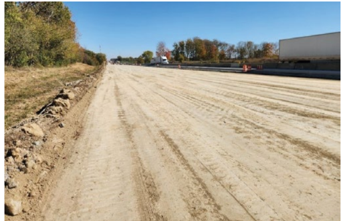
(a) Top of cement-treated subgrade layer on October 21, 2024, looking east from the west end of the project
