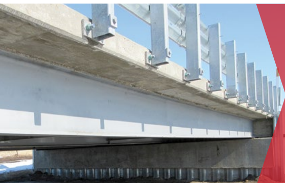
First bridge project in the US utilizing A709 Grade QST 65 steel: Buchanan County Sand Creek Bridge Project: Evaluation of the Performance of A709 Grade 65 QST Bridge Steel
