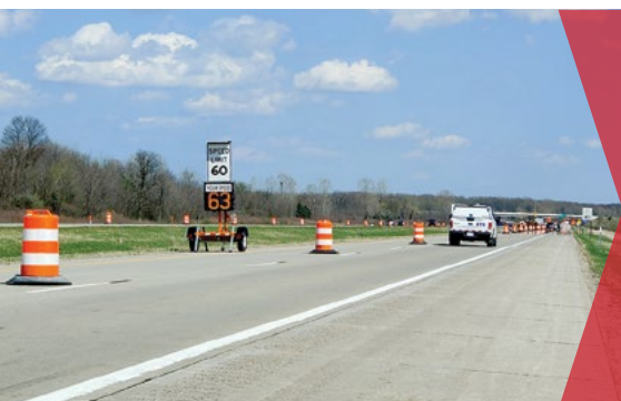
Speed feedback trailer positioned at the end of work zone lane closure taper Project: Work Zone Speed Limits and Motorist Compliance
