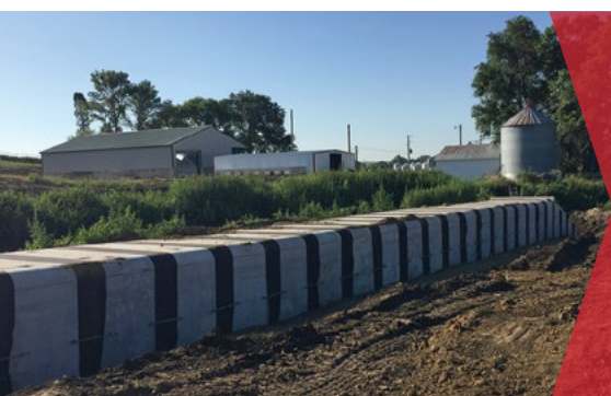
Culvert under construction showing precast concrete box sections in place Project: Concrete Box Culvert Earth Pressure Monitoring
