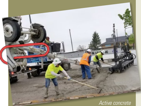
Active concrete overlay paving of a parking lot (Photo by City of Thornton, Colorado)
