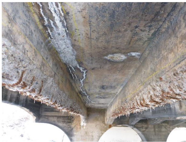
Figure 1. Spalling of concrete due to steel rebar corrosion
