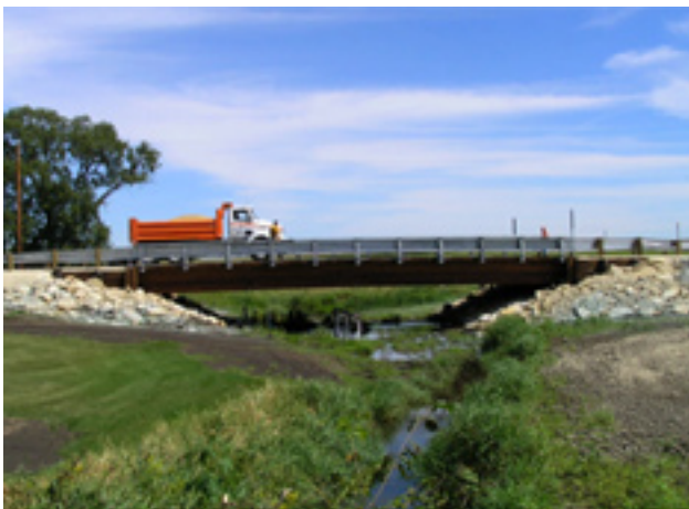
Bridge in Delaware County comprised of fiber-reinforced polymer (FRP), reinforced glued-laminated timber girders, and a transverse glued-laminated timber deck
