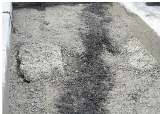
US Highway 422 in Indiana County, Pennsylvania, injected HDP foam into OGB under the pavement surface
