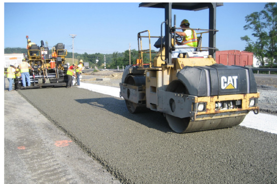
SR-22 near Clyde in Indiana County, Pennsylvania, construction of drainage ATB layer
