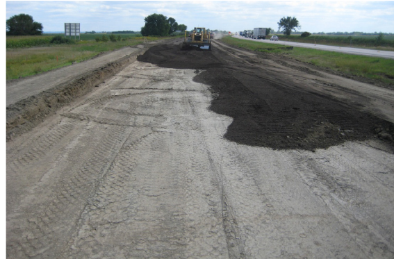
I-29 in Monona and Harrison Counties, Iowa, recycled pavement special backfill material over compacted subgrade
