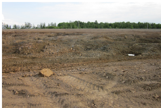
US Highway 10 just north of Junction City, Wisconsin, variable clay subgrade material
