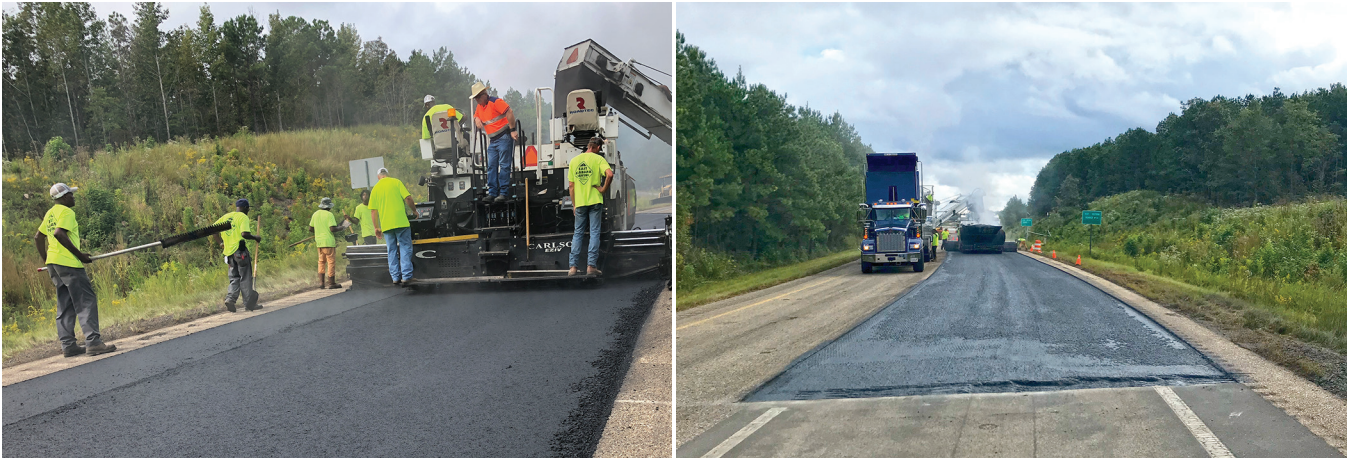
NCAT Test Track paving and compaction using first generation of BioMAG (biopolymer-modified asphalt mixture)
