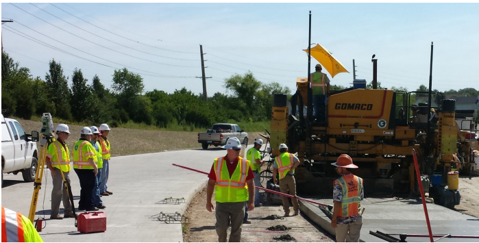
Figure 7. A total station pointing to a prism on the paving machine. Photo courtesy: Snyder & Associates, Inc.
