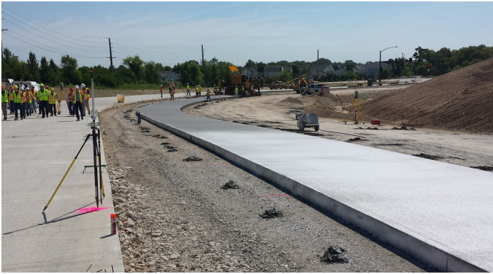
Figure 2. A stringless paving setup. No strings means better access for paving crews. Photo courtesy: Snyder & Associates, Inc.
